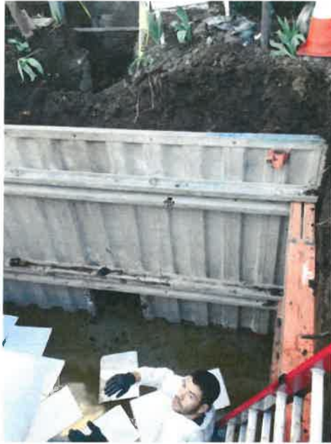
AREA OF BROKEN DELIVERY PIPING
