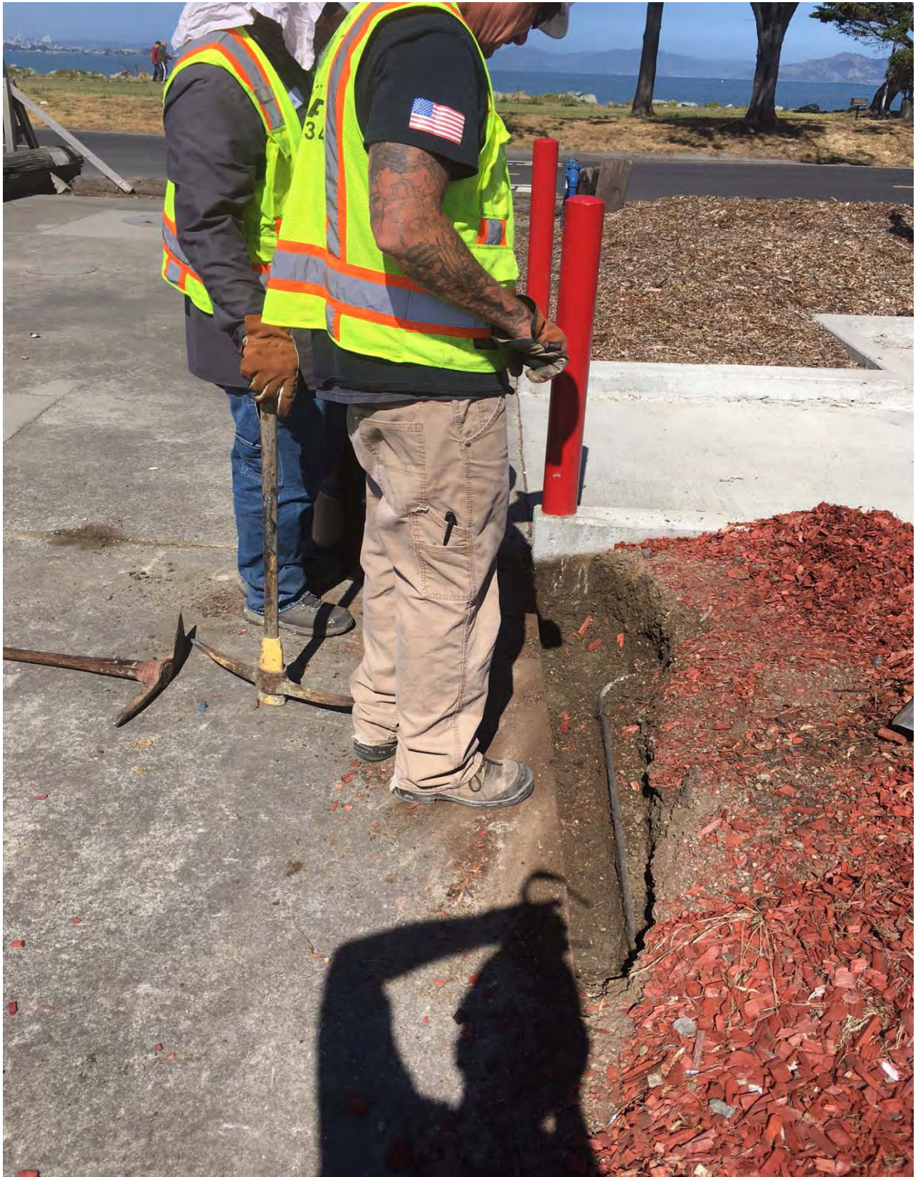
Excavation E-3 on north side of UST, note 2" conduit in sidewall at 18" bg
