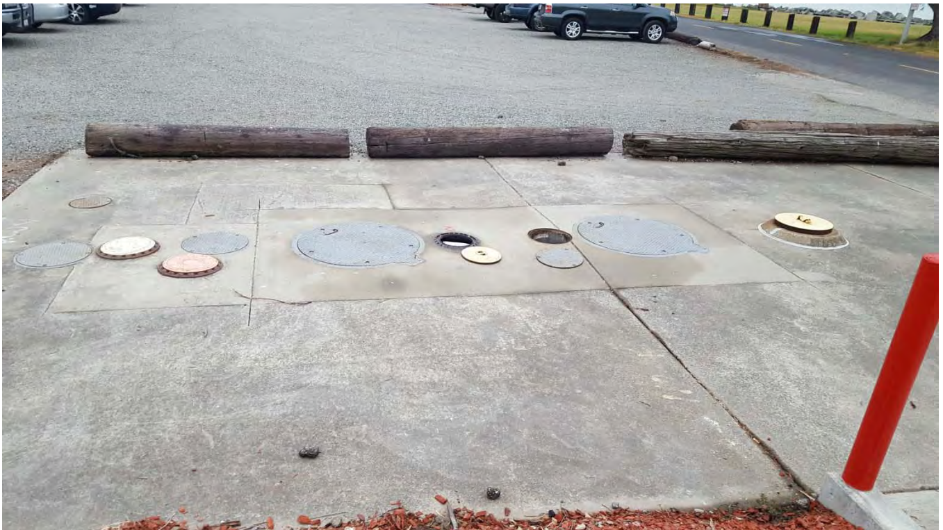
Note hydrocarbon stain in expansion joint leading off concrete pad
