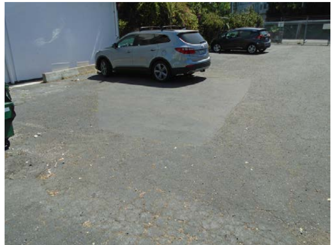
8. View of asphalt patch in northern portion of parking lot
