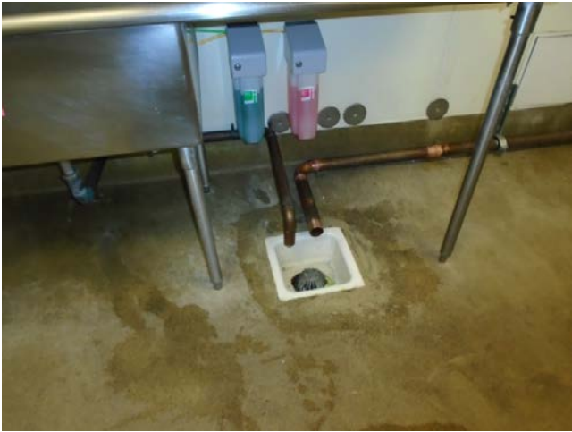
21. View of drain reportedly connected to grease trap, including typical staining
