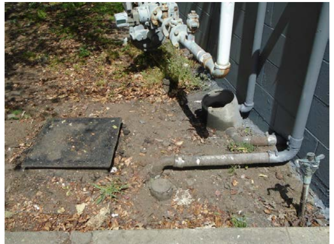
12. View of grease trap access point and grease staining on nearby utility features
