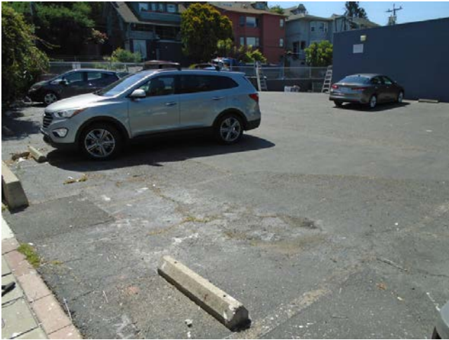
9. View of second asphalt patch in northern portion of parking lot
