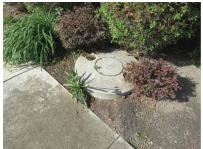
Picture 17 – Waste water sampling point
