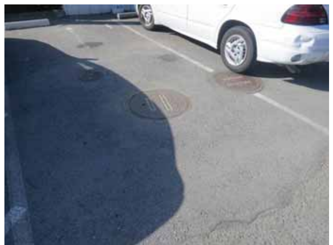
Picture 18 – Interceptor in parking area
