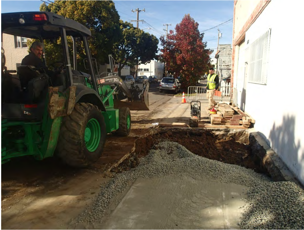
Backfill of excavation using clean overburden soil and clean import ¾" drain rock.
