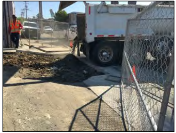
Photograph 16: Clean imported fill was also added to the UST pit to make up for the volume of the USTs.
