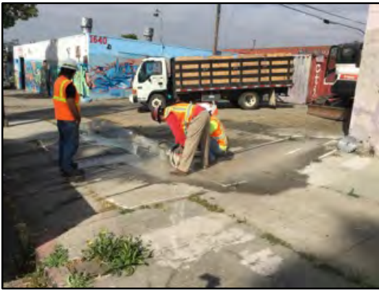
Photograph 1: A saw was used to cut the concrete slab above the third and fourth USTs. The excavation area had previously been cleared for utilities by USA.
