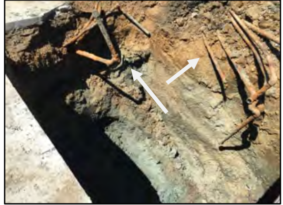
Photograph 14: Green staining was observed in the base and sidewalls of the fourth UST pit. Pipe lines were found running southwest towards the fifth UST and northwest into the subject property (arrows).
