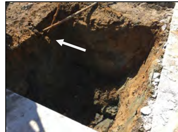
Photograph 6: Green staining was observed in the base and sidewalls of the third UST pit. Pipe lines were found running southwest towards the fourth UST (arrow).
