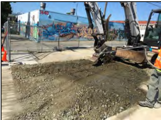
Photograph 17: The backfill was then compacted using a compactor wheel. Water was added to the soil during compaction for dust control.
