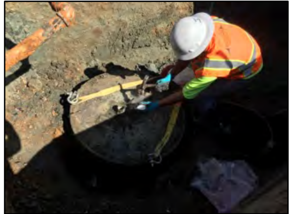
Photograph 10: Dry ice was added to the fourth UST to lower the oxygen level and Lower Explosive Levels (LELs).
