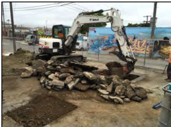
Photograph 29: Test pits were excavated to determine if other USTs existed on site. Test pit number 2 is shown at the bottom left corner and test pit number 3 is shown being excavated on the right.
