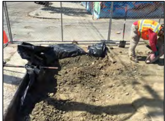
Photograph 24: The fifth UST pit was lined with a 6-MIL polyethylene liner before being temporarily backfilled with the stockpiled soil.
