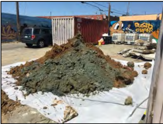
Photograph 3: Excavated soil was stockpiled on a 6-MIL polyethylene liner. Green hydrocarbon staining is visible in the stockpiled soil.
