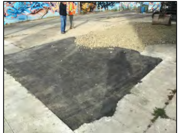
Photograph 18: The area above the third and fourth UST pit was temporarily asphalted over to match the existing grade.
