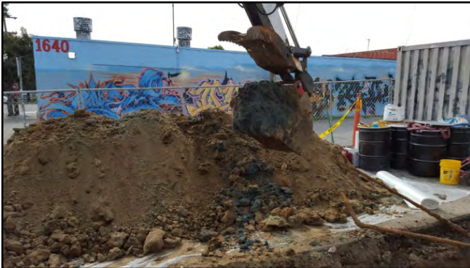
Photograph 3: Excavated soil was stockpiled on a plastic liner. Black hydrocarbon staining is visible in the stockpiled soil.
