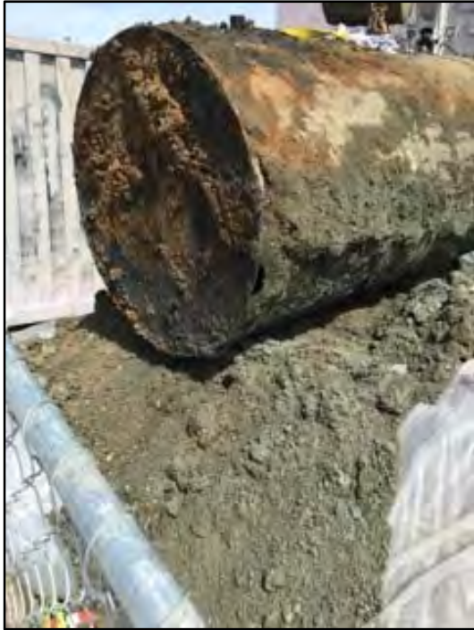
Photograph 11: Two holes were observed along the edge of the second tank.
