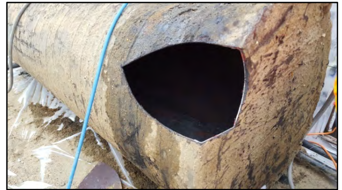
Photograph 6: A hole was cut into the side of the UST before it was hauled to Alco Iron & Metal Co. for disposal.
