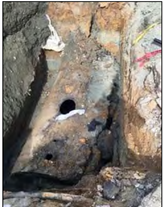
Photograph 10: The second UST in the tank pit just prior to removal. Olive green soil staining is visible at the base of the pit.
