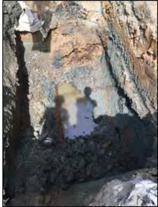
Photograph 12: Water encountered at the base of the UST pit was sampled. The water, located at the portion of the pit where the UST had rested, may have been rinsate that leaked from the tank. No water was observed in areas of the pit that had been excavated to a deeper depth.
