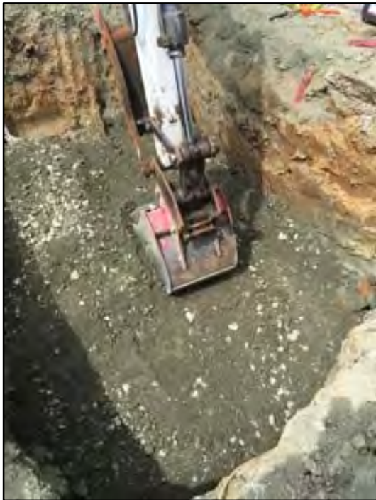
Photograph 13: The excavator bucket was used to compact the backfill in the tank pit in 2 ft increments.
