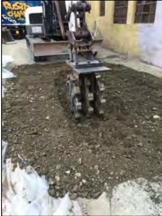
Photograph 15: A compactor wheel was used to compact the surface of the backfill.
