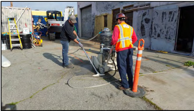
Photograph 1: A saw was used to cut the concrete slab above the first UST. The excavation area had previously been cleared for utilities by USA.
