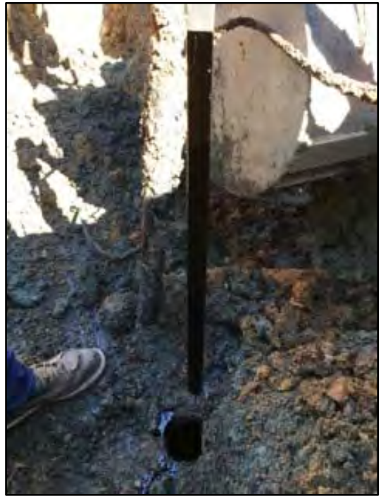
Photograph 8: A PVC pipe was used to determine the thickness of the fuel oil present in the second tank before pumping out the contents.
