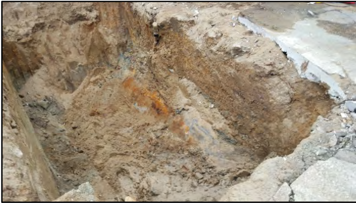
Photograph 7: A second UST was discovered beneath and adjacent to the first UST. The UST fill pipe can be seen above the rusty brown area of the tank.
