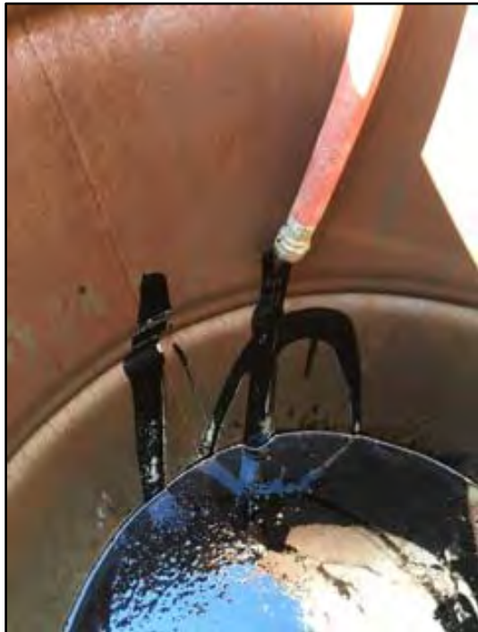
Photograph 9: The tank contents were pumped into 55-gallon drums. The drums were stored on-site pending waste characterization.
