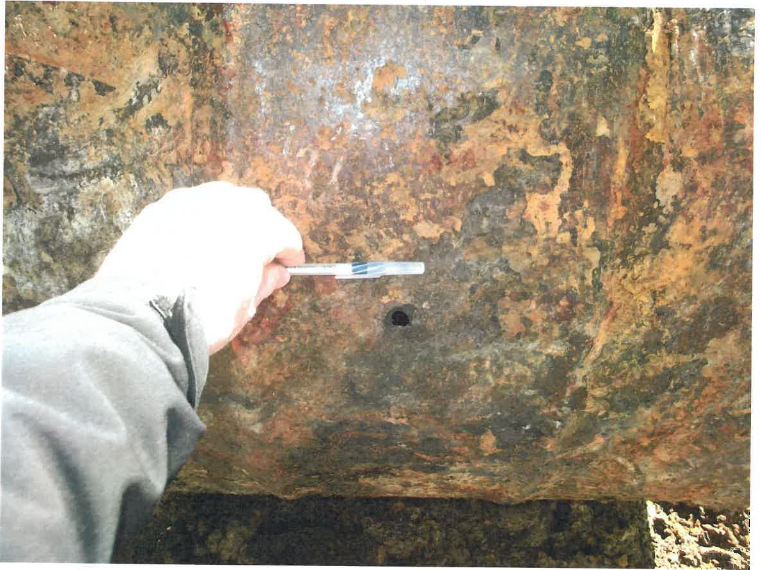
Image #3 Close-up of hole on north side in upper half on west half of UST.
