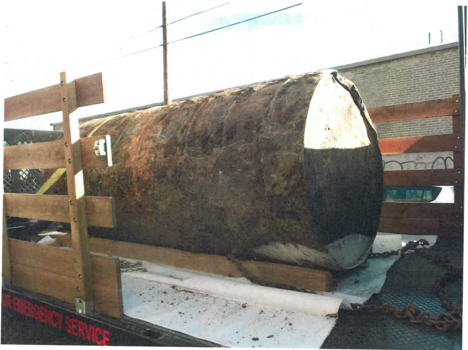
Image #5 UST on truck for transportation.
