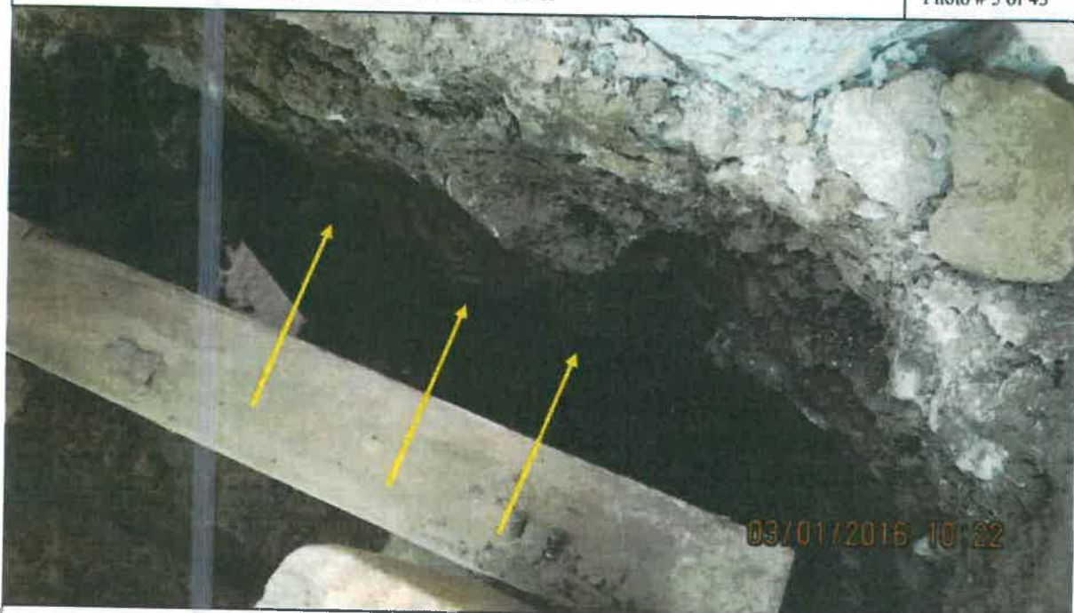
DESCRIPTION: VIEW OF WHAT IS BELIEVED TO BE PRODUCT, RETURN, AND VENT PIPING
