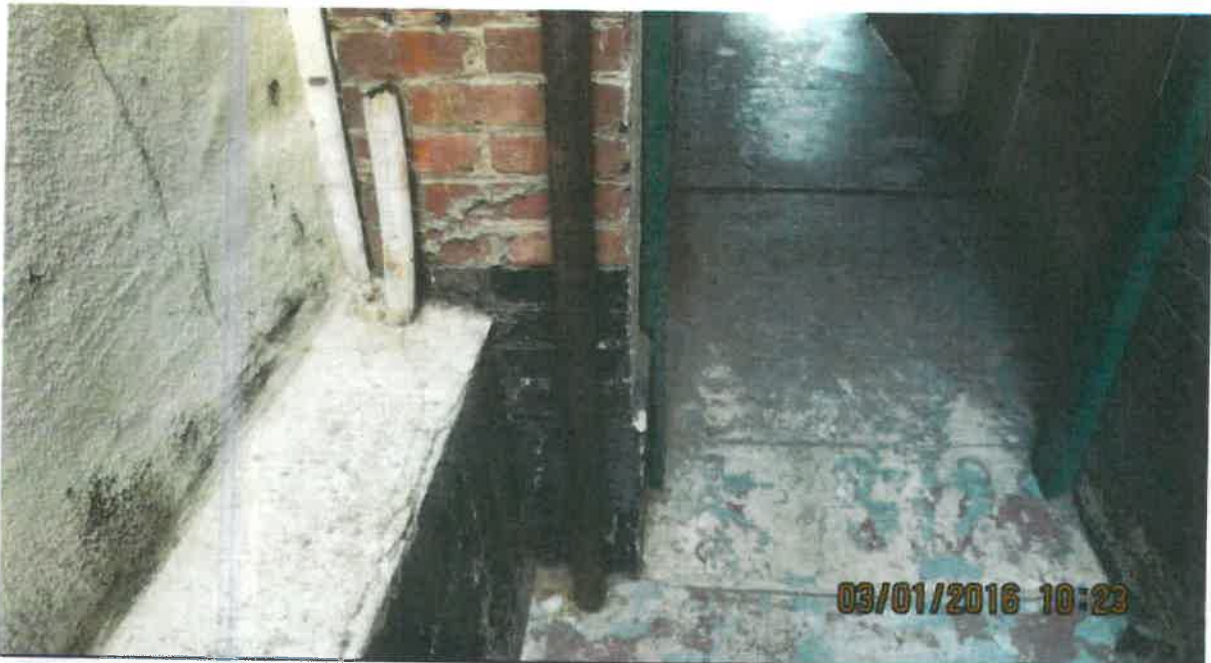
DESCRIPTION: VENT PIPE
