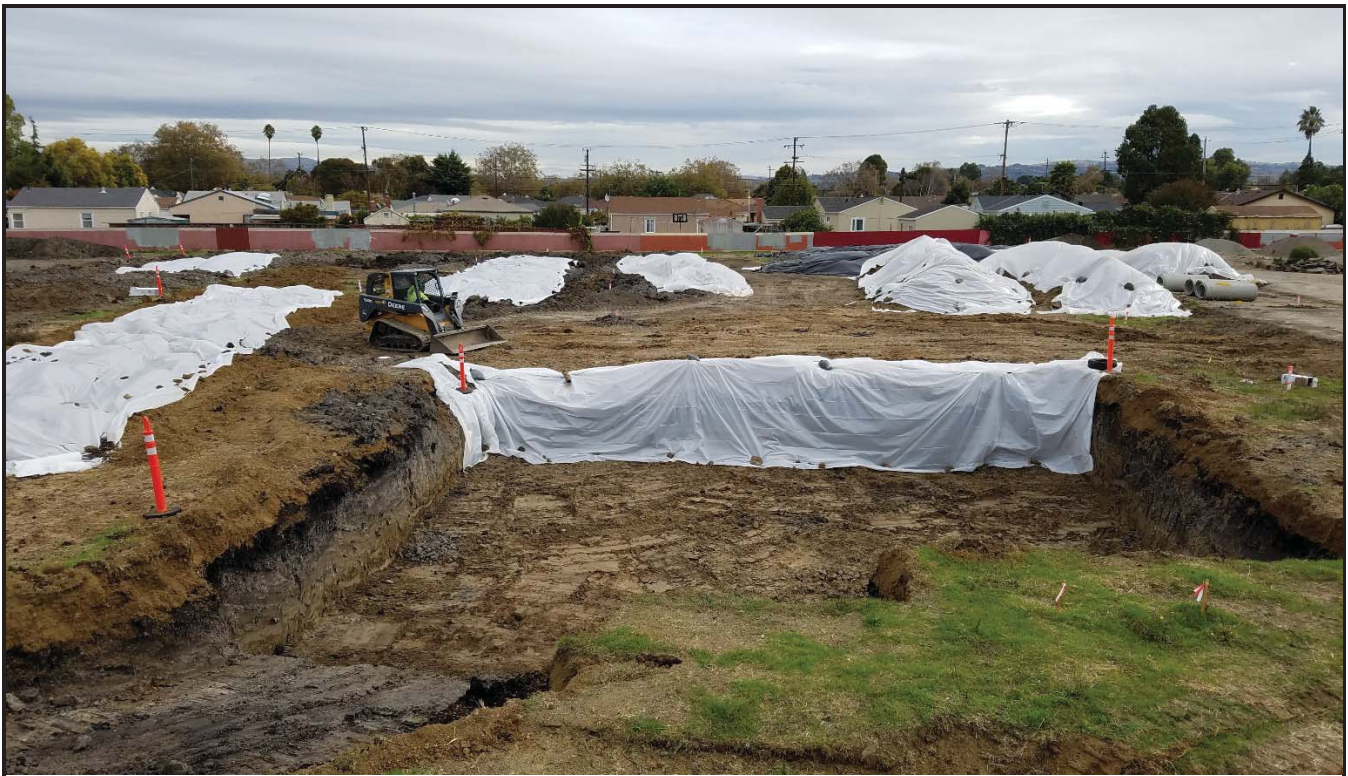
Photo 2. PTN excavation area with plastic vapor barrier along east sidewall and covered stockpiles
