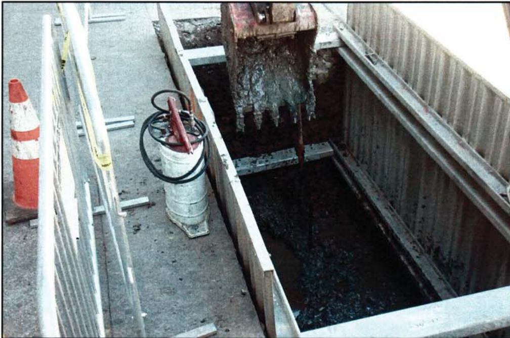
Groundwater in Excavation
