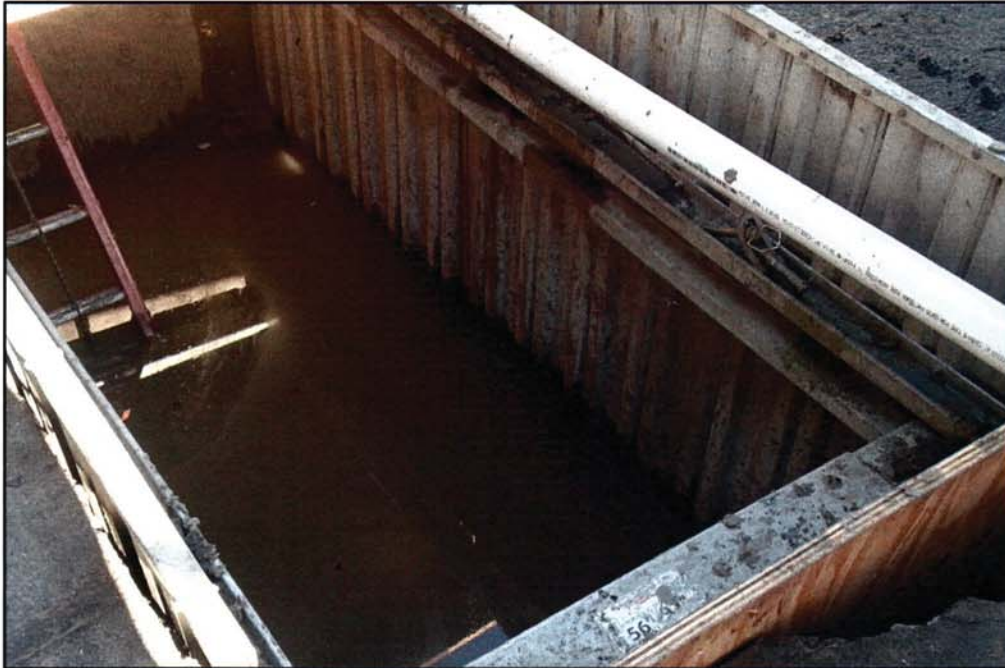
Groundwater in excavation.
