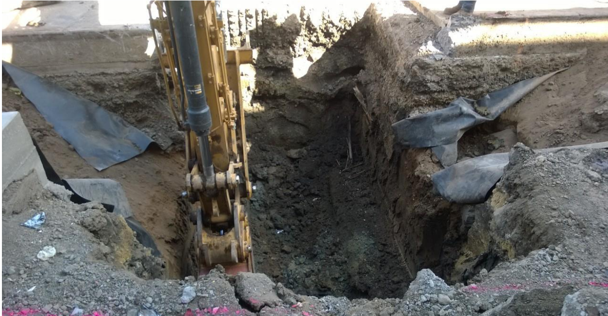
DESCRIPTION: SOIL SAMPLE COLLECTED FROM WEST SIDE OF EXCAVATION AT SIDE WALL OF TANK
