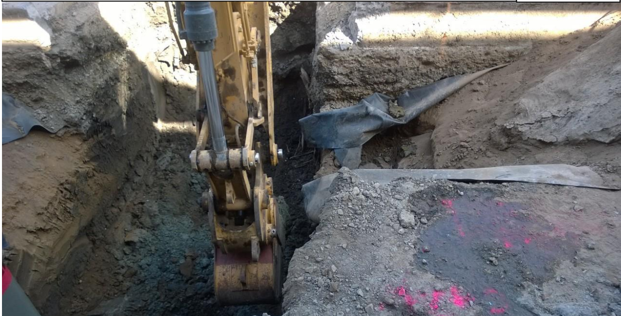
DESCRIPTION: SOIL SAMPLE COLLECTED FROM EAST SIDE OF EXCAVATION AT SIDE WALL OF TANK
