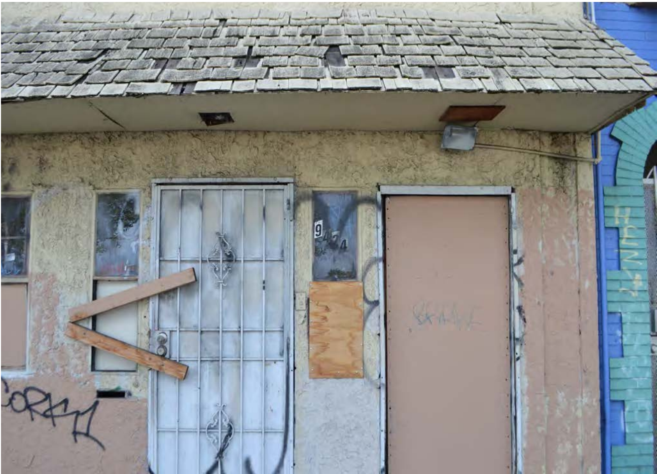
Photo 5: Dilapidated property at 9424 apartment units in very poor condition
