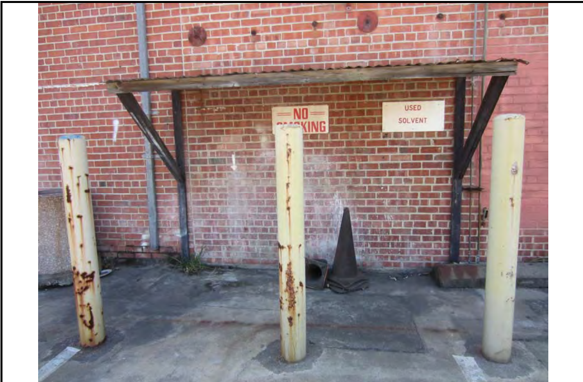
Photograph: 3 | View of former solvent storage at the western exterior of Building 1.
