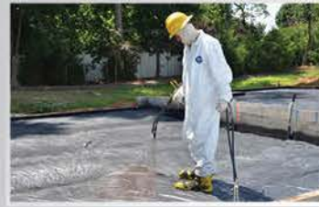
Geo-Seal CORE is spray applied to increase the systems tensile strength and provide a seamless membrane
