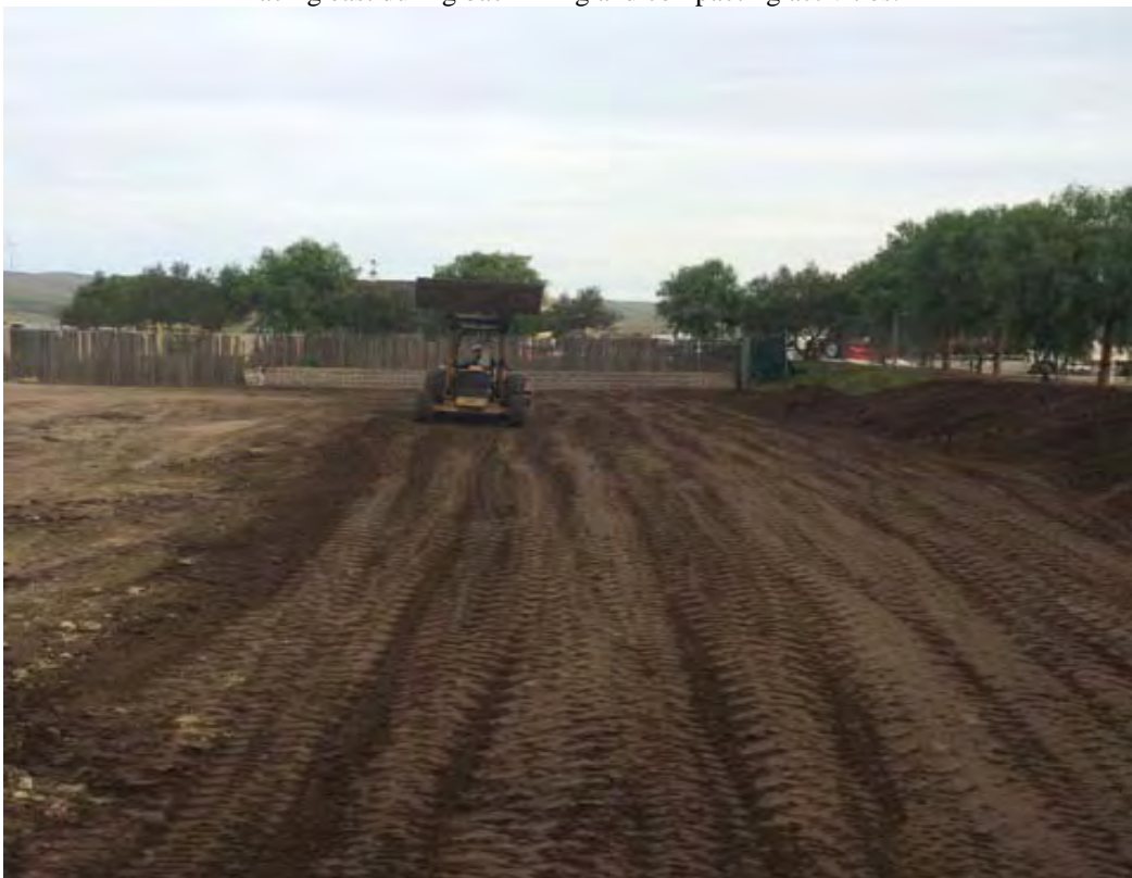
Photograph 4: Facing east from the western edge of the excavation as backfilling complete.
