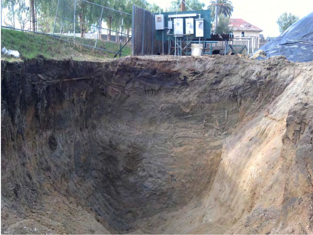
Photograph 1: Facing westerly at the final excavation western wall next to electrical power.
