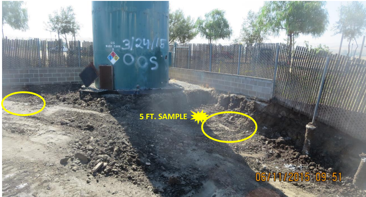
DESCRIPTION: SOUTHEAST VIEW OF EXCAVATION HOLE - & ESTIMATED LOCATIONS OF TWO TANKS REMOVED – ESTIMATED SOIL SAMPLE LOCATION
