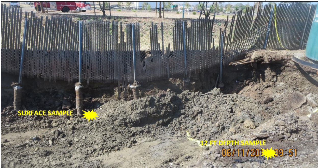
DESCRIPTION: VIEW OF EXCAVATION HOLE – ESTIMATED SAMPLING LOCATIONS AND DEPTHS ACCORDING TO FACILITY
