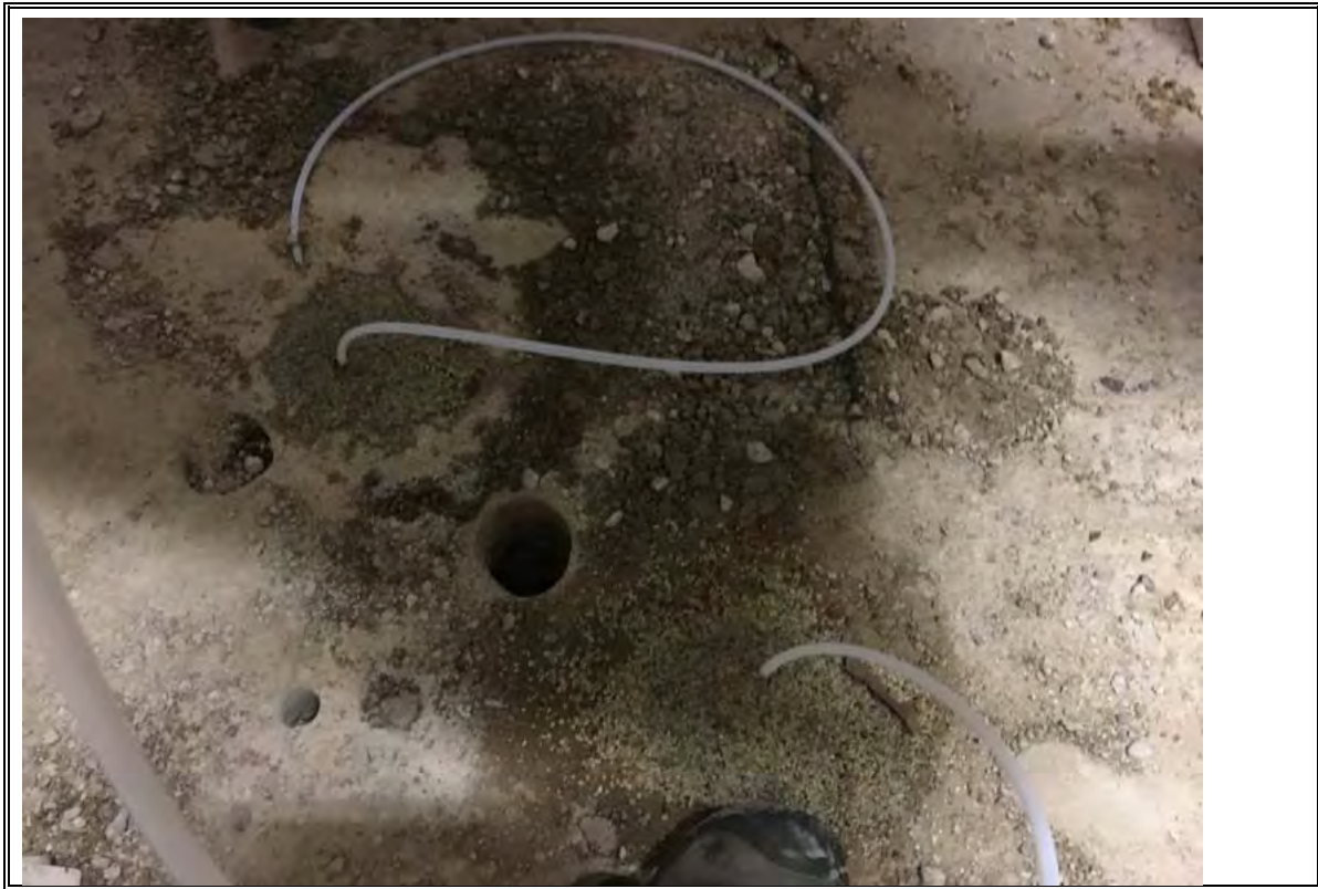
5. SV-1-3 and SV-1-5 in the utility room.
