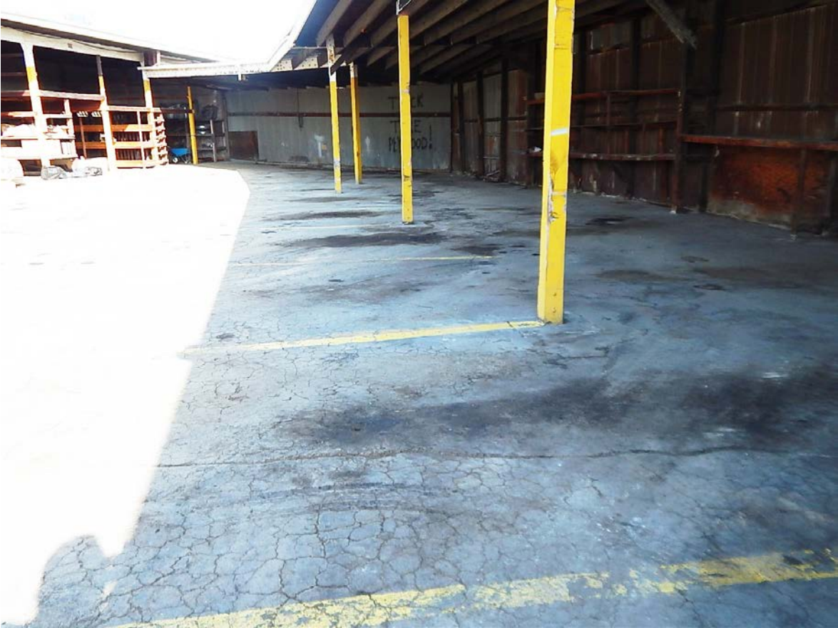
Photograph 8 - View of interior of the shed area with oil stained asphalt
