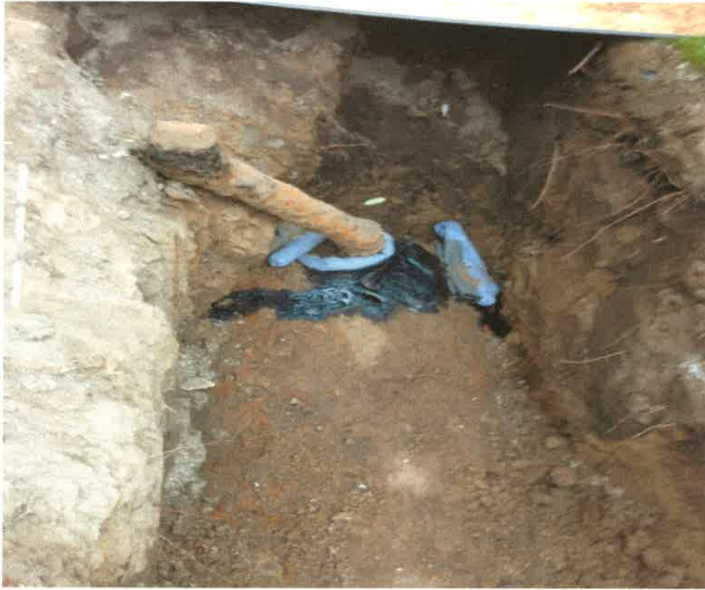
Main fill pipe. Product seepage is visible on surface of the tank
