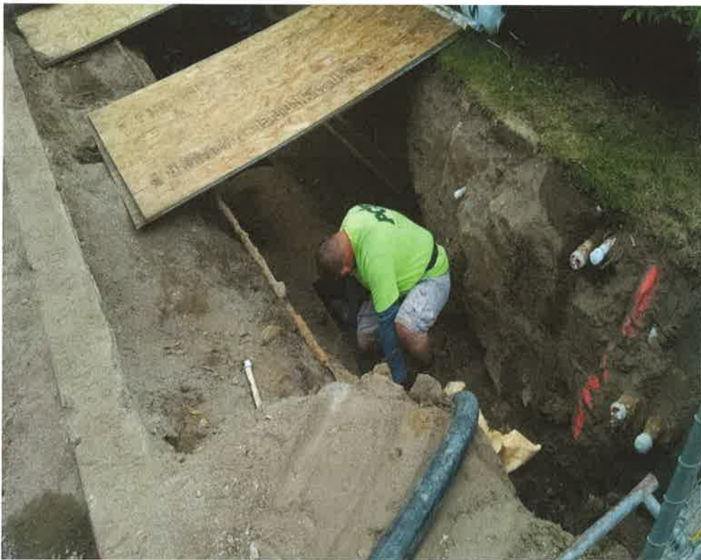
Pressure filling tank with CDF
