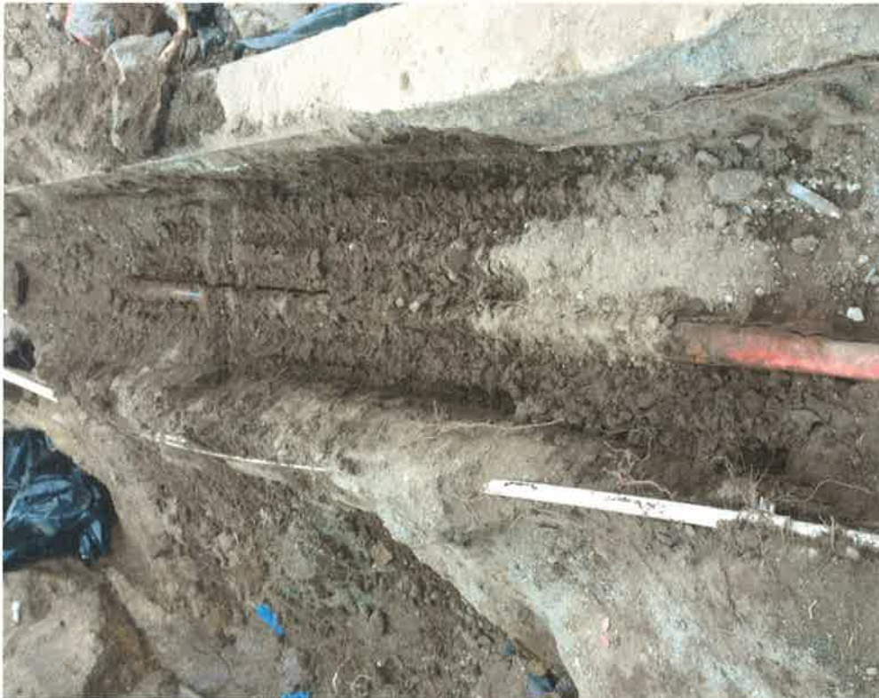
Photograph of return line found running parallel to North edge of tank
