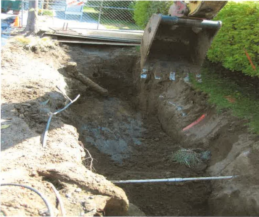
UST excavation facing east. The main fill pipe is visible in the background
