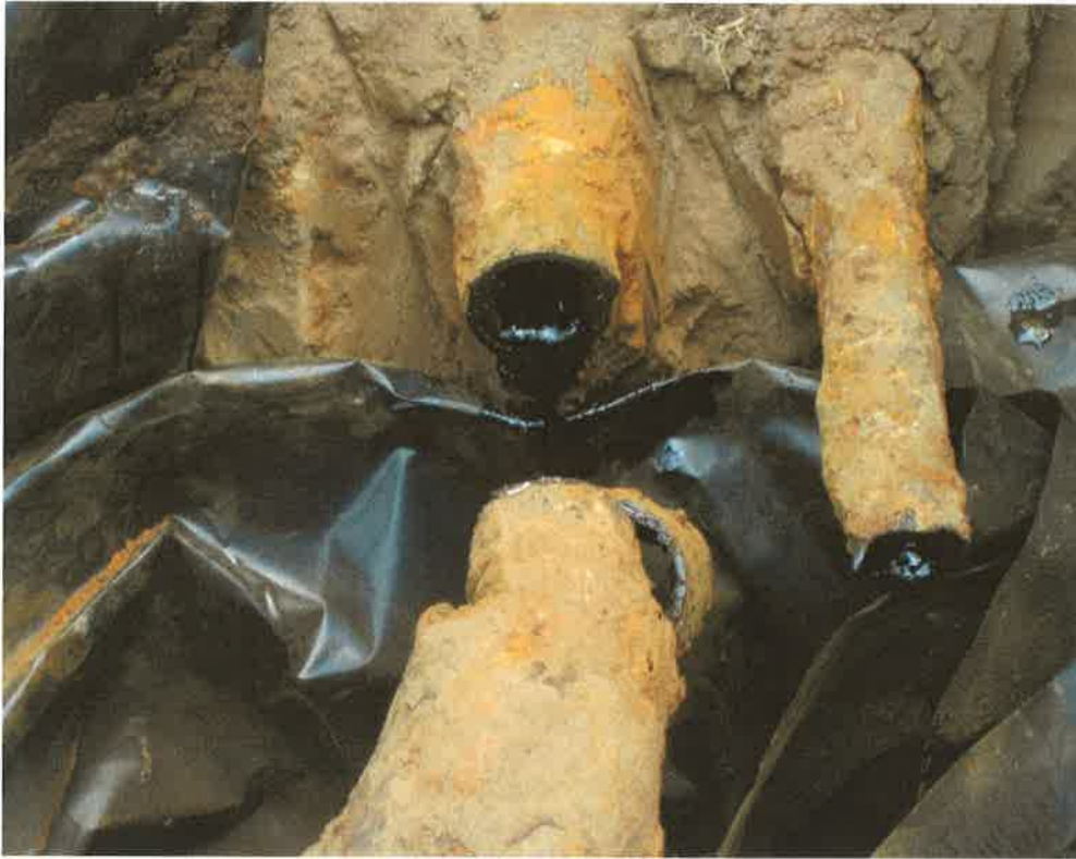
Photograph showing product seeping from pipes
