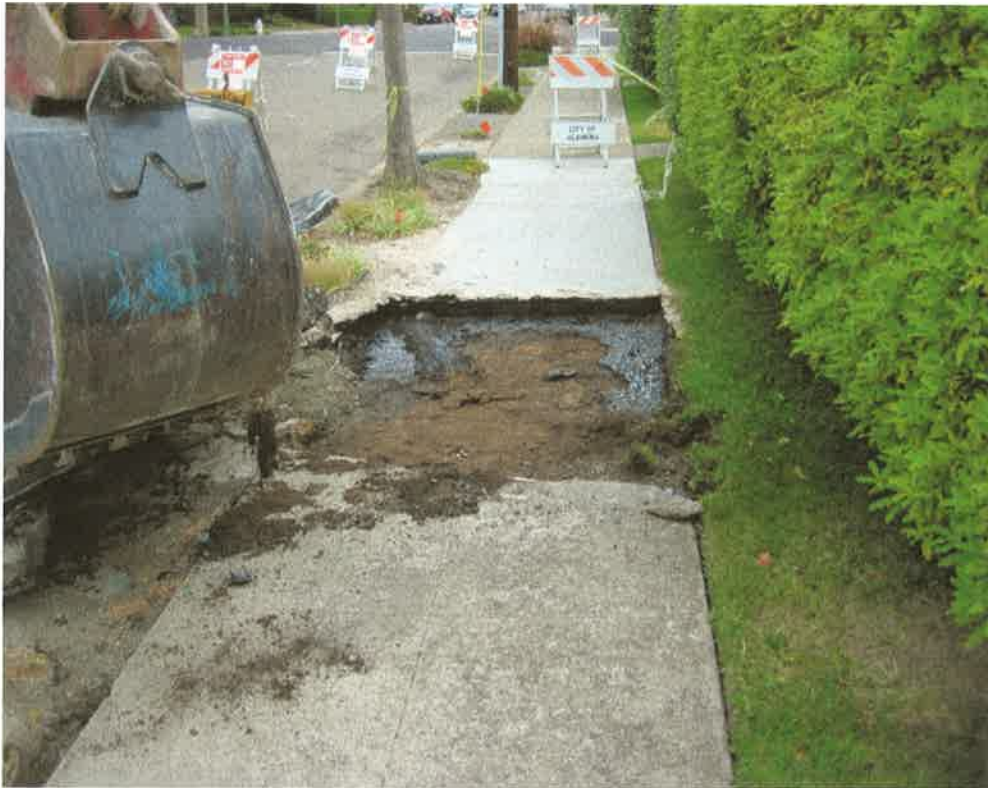
Photograph showing oil product seep beneath the sidewalk
