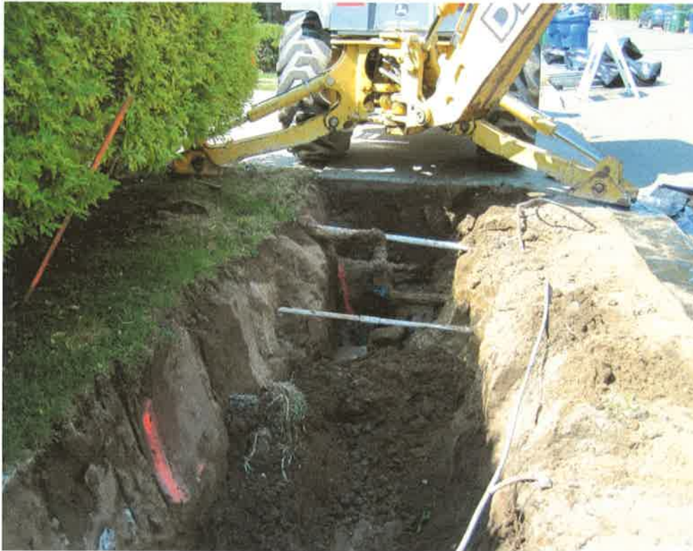
UST excavation facing west. The product delivery system manifold and piping is visible in the background
