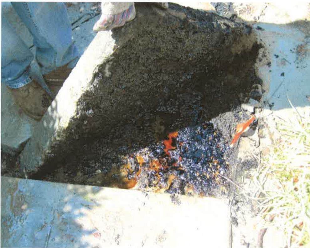
Additional photograph showing oil seep beneath sidewalk
