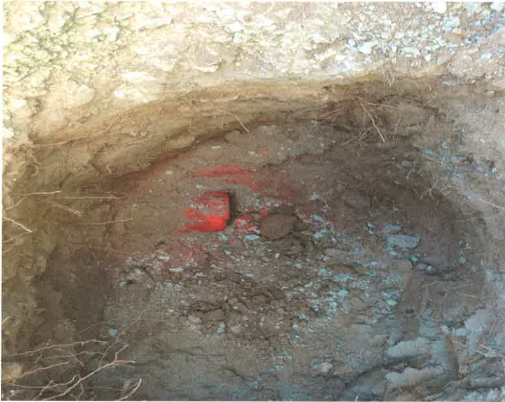
Termination point of return line found at utility pole
