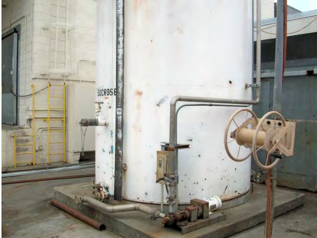
19. View north of location of empty sucrose AST at southwest end of service area.
