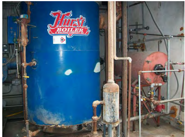
16. View of package boiler unit and expansion tank in service area.
