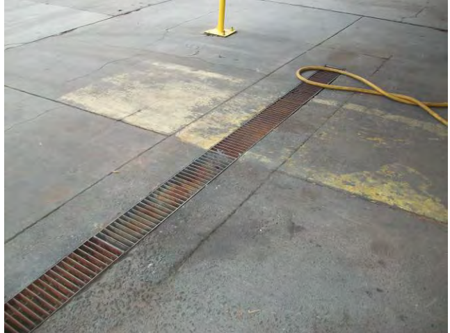
8. View of storm water drain in driveway along southwest side of Building 1.
