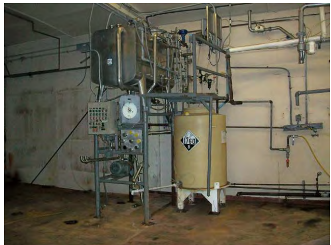
6. View of Building 1 idle food processing equipment and empty sanitizing chemical AST.
