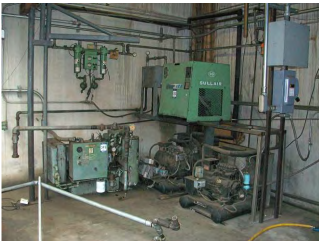
17. View of air compressor units in service area.
