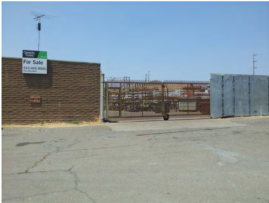
Ph-12 Side Gate in front of Concrete Patch associated with UST Removal
