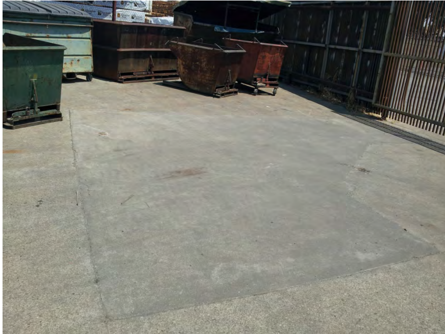
Ph-11 Concrete Patch where USTs were supposedly Removed
