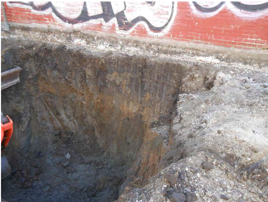
Photo 6 Note Contaminated Soil Left in Place Beneath Foundation of Adjacent Building
