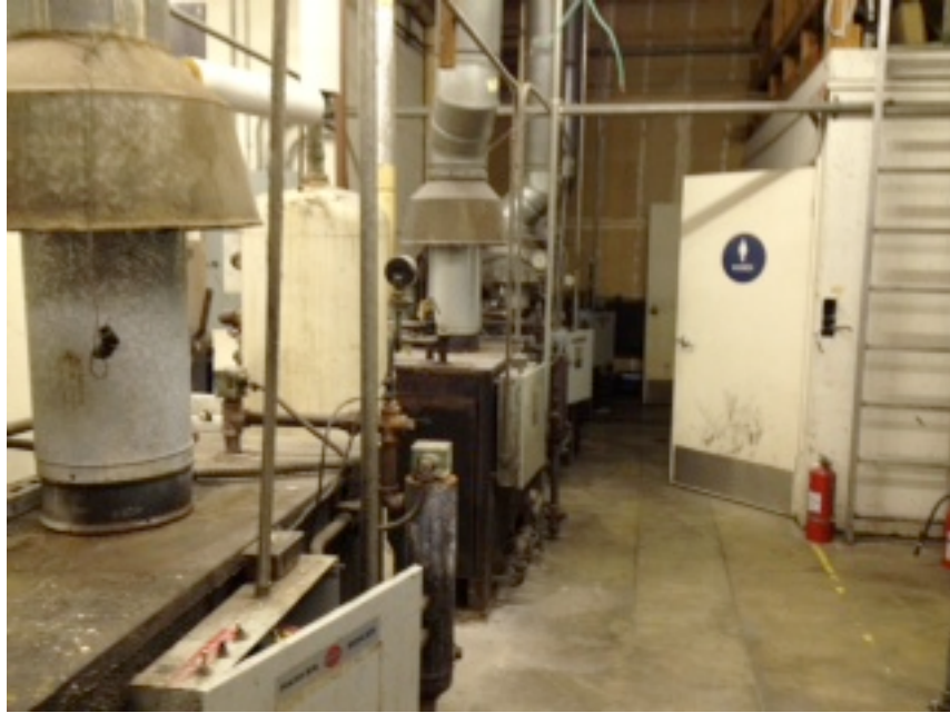
Photo 15: Boilers in Storage Hallway (Facing East) 7104 Dublin Blvd
