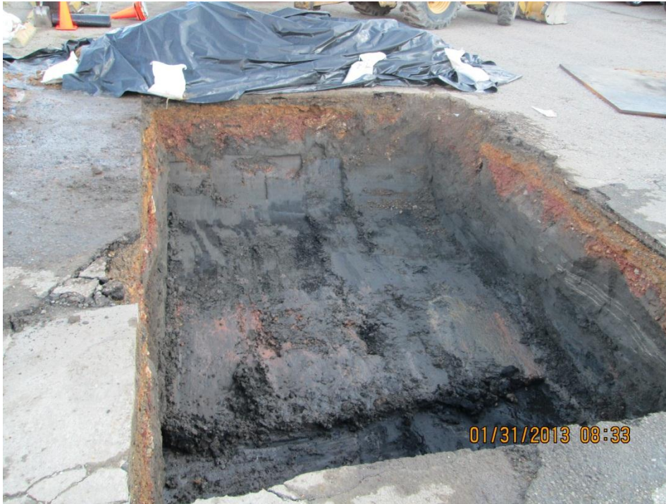
Photograph 1. View of excavation on January 31, 2013 after ponded water had been pumped from the excavation.
