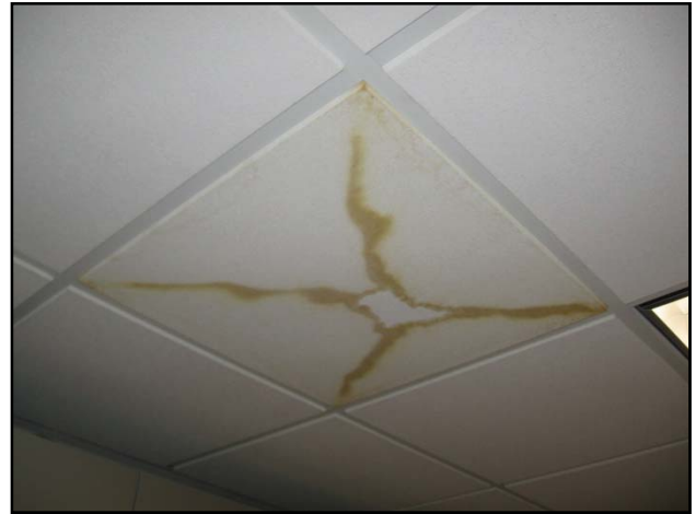
Photograph 8: Stains were observed on ceiling tiles on the upper level of the northern tenant space. The stains could have been caused by a leaking roof or pipe, or by an air-conditioning (condensation) leak.
