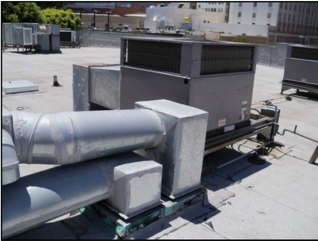
Photograph 7: Heating and air conditioning for the building is provided by a packaged HVAC unit on the roof. The roofing material appears to be in good condition, but has some patching compound around a few vent pipes.
