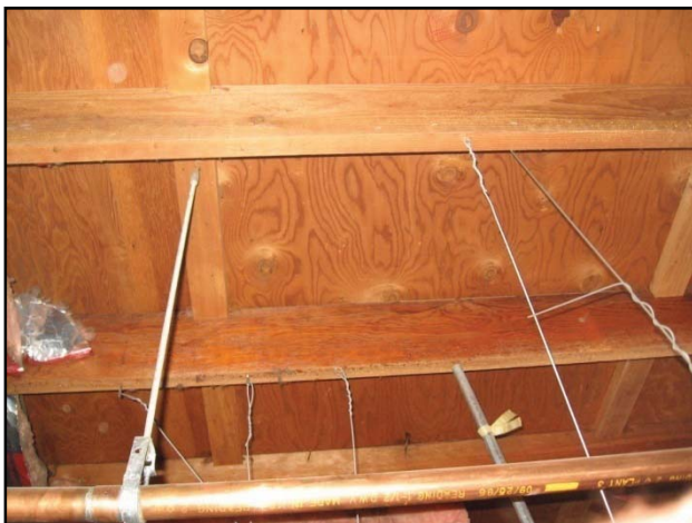
Photograph 5: The roof is constructed out of glue-lam beams with interstitial wood joists. Fiberglass insulation was observed above suspended ceiling tiles; the wood-framed portion of the roof has no insulation.
