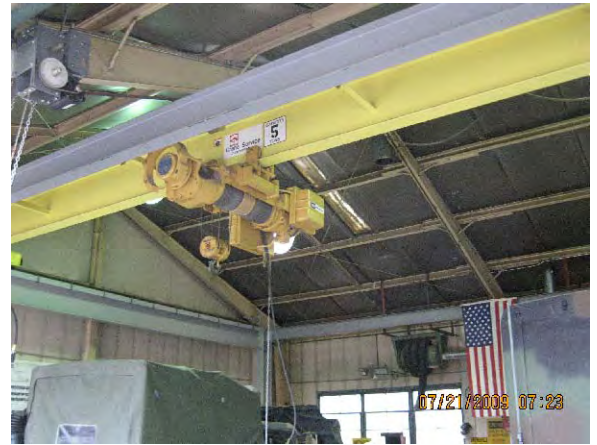
PHOTOGRAPH 8. Overhead crane used to lift vehicles for maintenance. Hydraulic lifts not installed.
