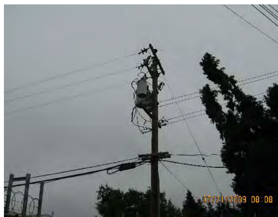
PHOTOGRAPH 4. Overhead transformers located along southern boundary of site.
