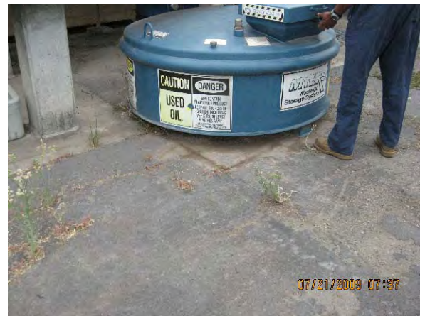
PHOTOGRAPH 10. Used motor oil AST. Area beneath AST contained absorbent material. Staining around AST minimal.
