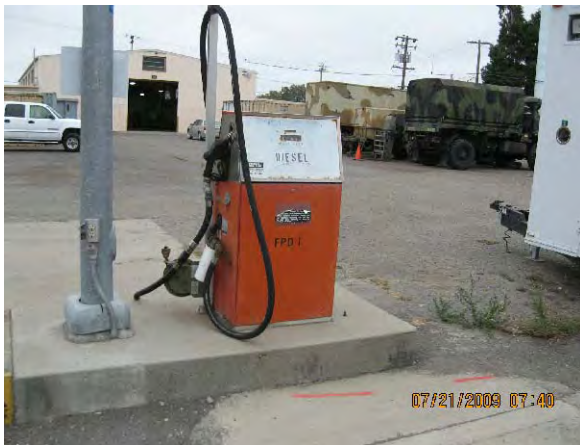
PHOTOGRAPH 9. Diesel fueling pump, located north of maintenance building.
