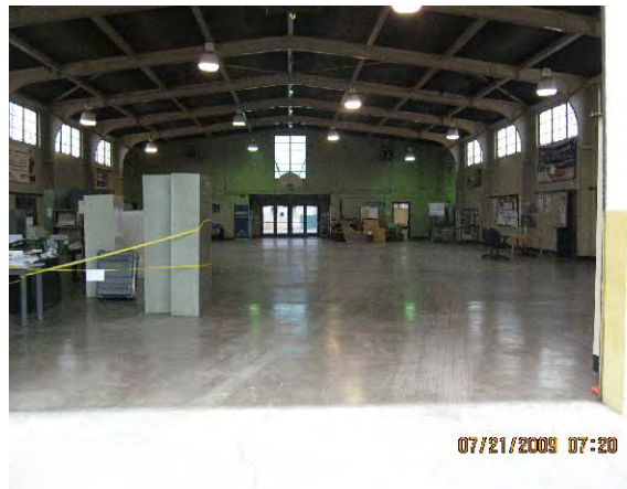
PHOTOGRAPH 2. Interior view of main room of armory building, with office doors visible along the edges. Stored furniture appeared to have been removed to allow asbestos abatement of select rooms.
