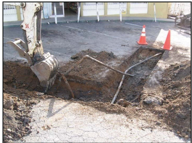
Photograph 4: Piping detected during the geophysical survey at the central portion of the parking lot was excavated using a Bobcat and removed. Soil samples were collected from beneath the pipe openings and joints.
