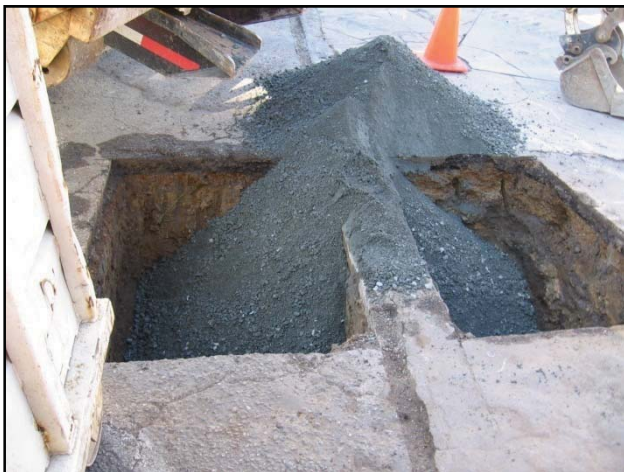
Photograph 5: The excavations were filled with clean, imported Class II AB fill material.
