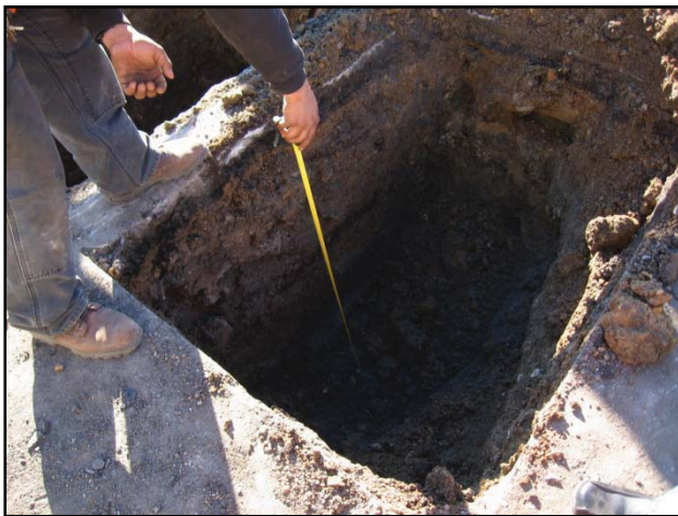
Photograph 3: A pit excavated to 5 ft bgs at the southeast parking area was at the location of an anomaly detected during a previous geophysical survey. The electrical line running through the middle of the excavation was not disturbed.
