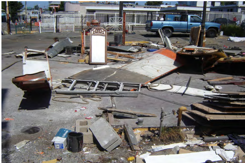
9. A second picture of building debris.
