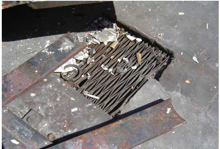
11. A picture of the drain located on the subject property, next to the hydraulic lift.
