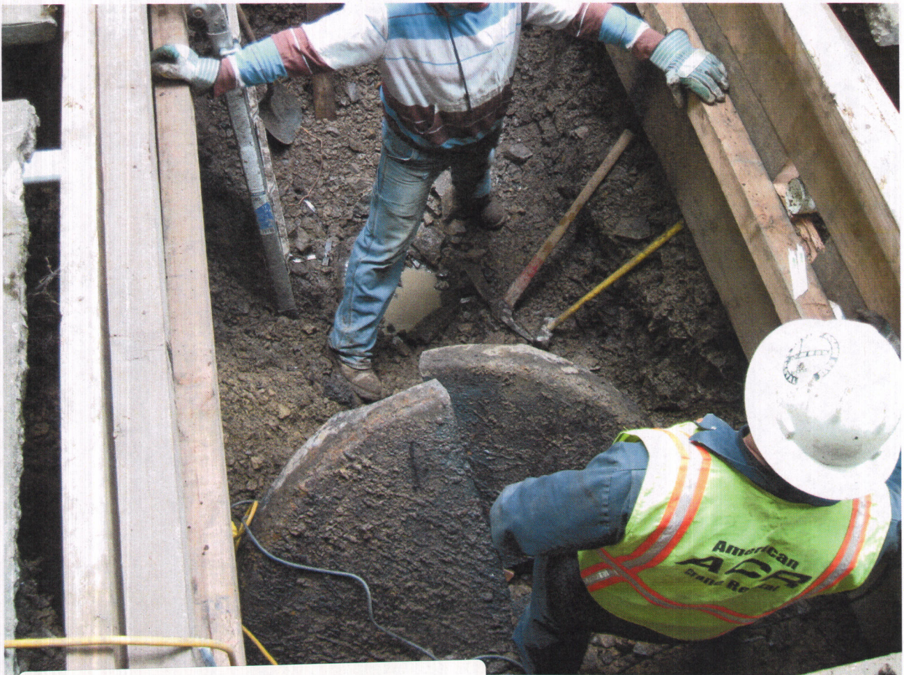
40 Crocker Avenue Piedmont CA 94611 RWeston 4-13-2010 Single wall steel (heating oil tank) two soil piles, tank removed in pieces
