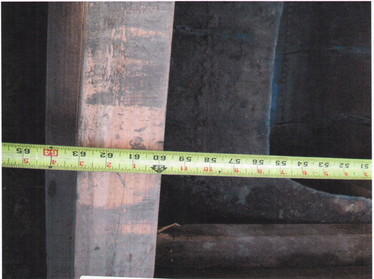
40 Crocker Avenue Piedmont CA 94611 RWeston 4-13-2010 Single wall steel (heating oil tank) tank 5' diameter, 8' to bottom of tank
