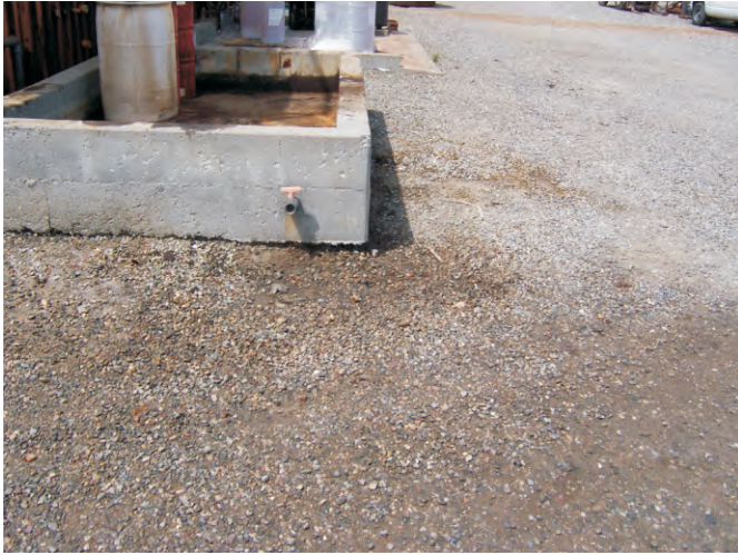
Photograph 7: Stained gravel adjacent to secondary containment (View to the southwest).
