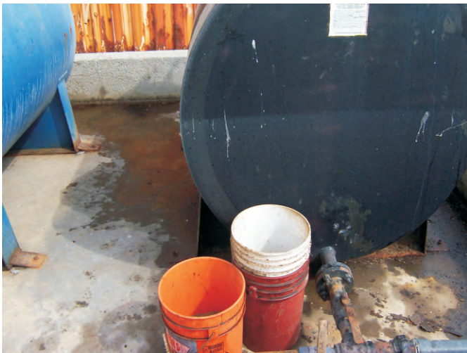
Photograph 3: Visible oil and staining within concrete secondary containment (View to the north).
