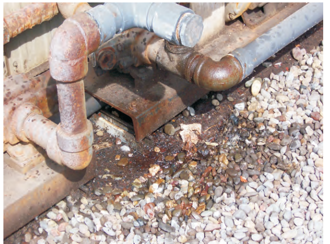
Photograph 4: Visible oil on gravel, adjacent to southeast side of building (View to the west).
