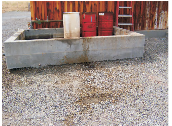
Photograph 6: Stained gravel adjacent to secondary containment (View to the southeast).
