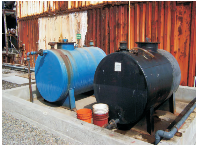
Photograph 2: Two AST's used for new and used oil (View to the northwest).
