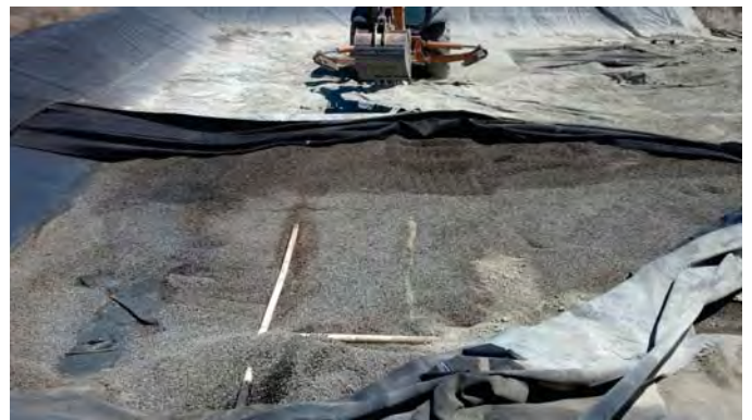
Photograph 4: Exposing Lysimeter in Base Gravel Separating Primary and Secondary Liners (View to the North).
