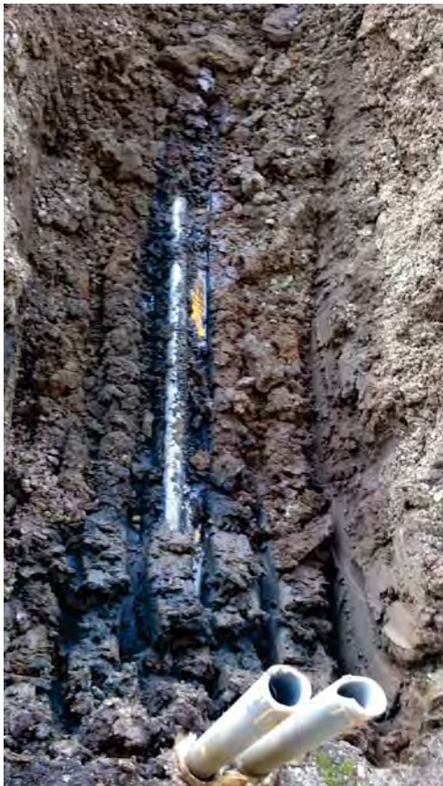
Photograph 7: Excavation Between Evaporator Pads #2 & #3. Note Soil Staining Along Conduit Runs (View to the east).
