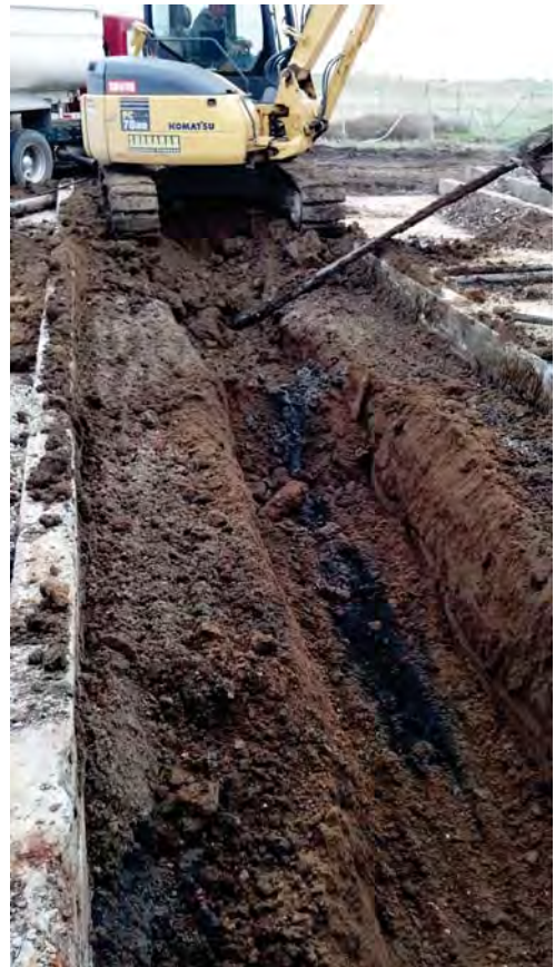
Photograph 8: Excavation Between Evaporator Pads #2 & #3. Note Soil Staining Along Conduit Runs (View to the east).
