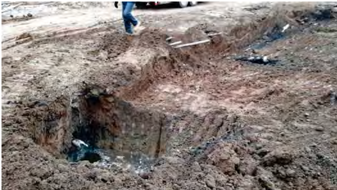
Photograph 15: Soil Staining Along Conduit Trenches (View to the southeast).
