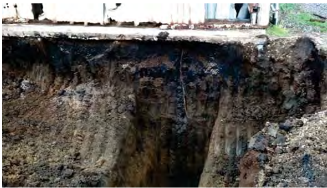
Photograph 19: Excavation at the Northeast Corner of the Building (View to the west).
