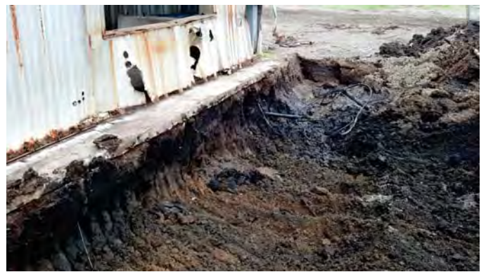
Photograph 20: Excavation at the West-end of Evaporator Pad #5 at the Northeast Corner of the Building (View to the northwest).
