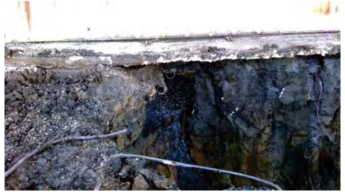
Photograph 12: Electrical Conduits at Southeast Corner of Building. Note Free-Phase Fluid in Conduit Trench (View to the west).
