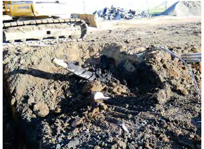
Photograph 14: Soil Staining Along Conduit Trenches (View to the southeast).
