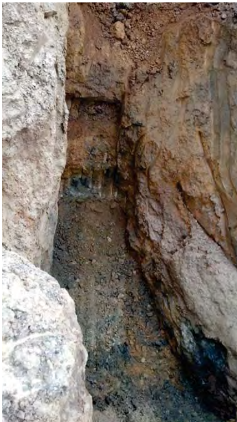
Photograph 31: Deep Excavation (~18 feet bgs) of Impacted Soil Beneath Piping "T" Connection Near East -end of Evaporator Pads #3 & 4 (View to the south).
