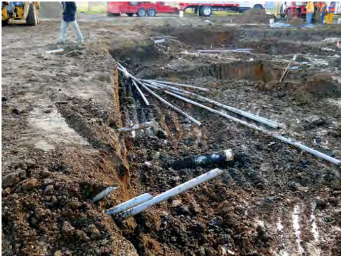
Photograph 13: Soil Staining Along Conduit Trenches (View to the south).
