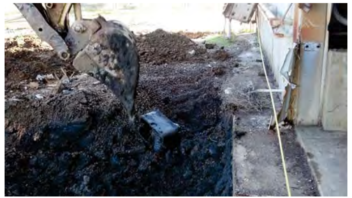
Photograph 18: Building Ground Rod Box Adjacent/South of Evaporator Pad #1 Containing Free-Phase Product (View to the south).
