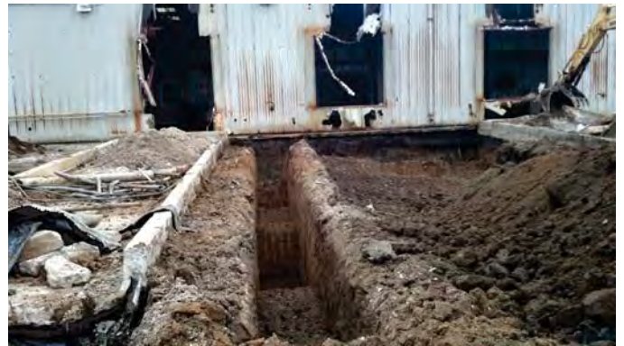
Photograph 26: Excavation of Soil Impacts related to Conduit Trench Between Evaporator Pads #1 & 2 (View to the west).
