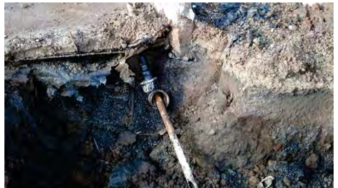
Photograph 10: Excavation of Secondarily Contained Piping at Northeast Corner of Evaporator Pad #1. Note Soil Staining Around Piping (View to the west).
