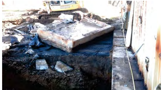
Photograph 22: Removal of Evaporator Pad #1. Note Gravel Base is Saturated with Free-Phase Product (View to the south).
