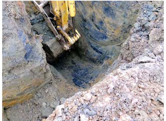
Photograph 28: Deep Excavation (~18 feet bgs) of Impacted Soil Beneath Piping "T" Connection Near East-end of Evaporator Pads #3 & 4 (View to the southeast).
