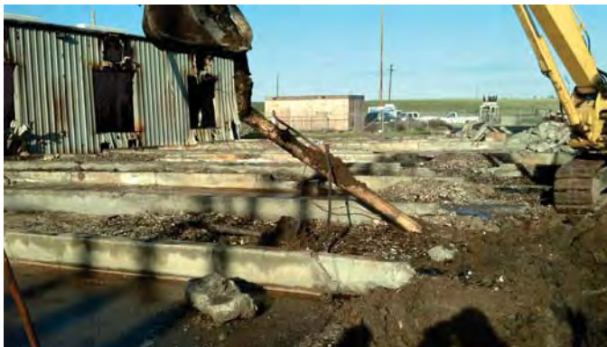
Photograph 9: Excavation of Secondarily Contained Piping at Northeast Corner of Evaporator Pad #1 (View to the northwest).
