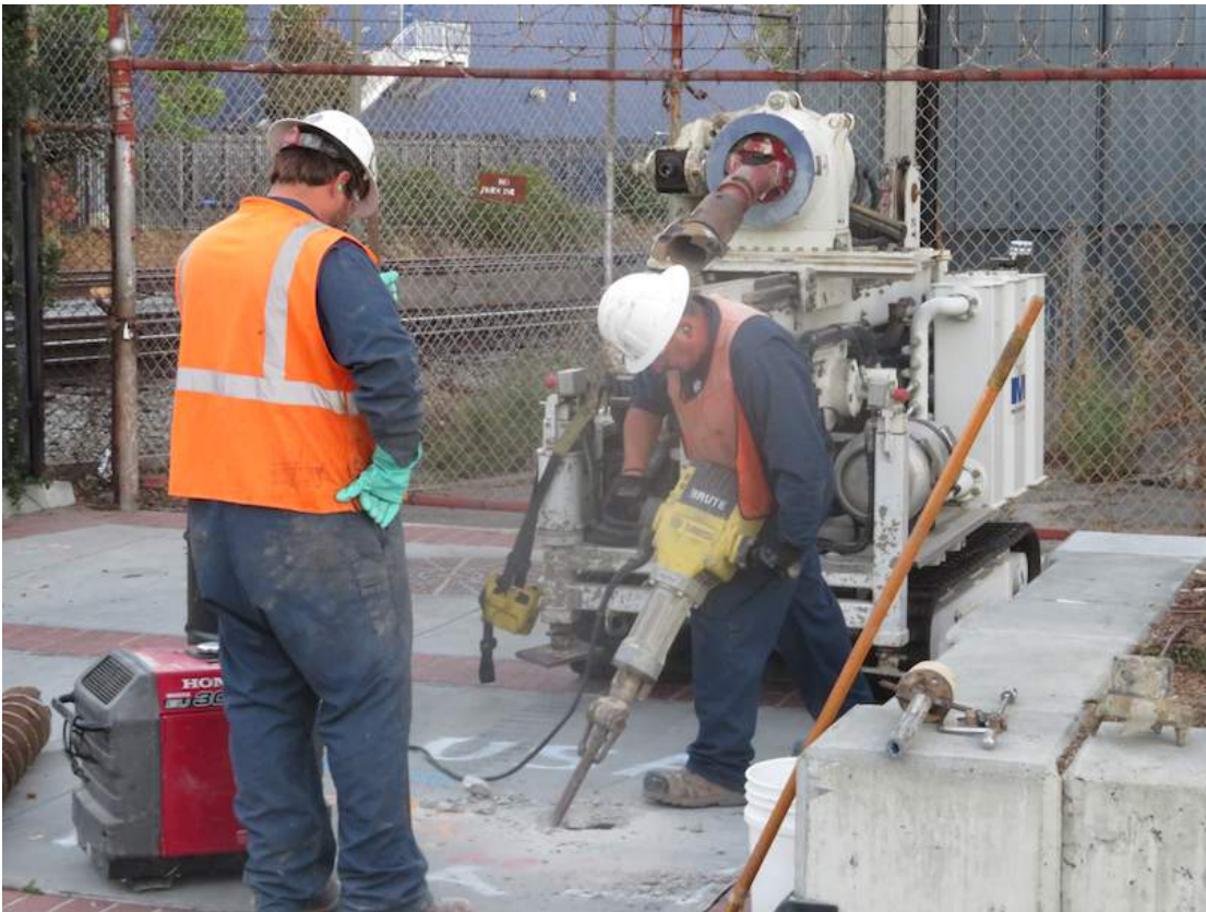
Photograph 2 – Using jack hammer to clear well head from surrounding concrete. Jack hammer is powered by generator in left bottom of photo.
