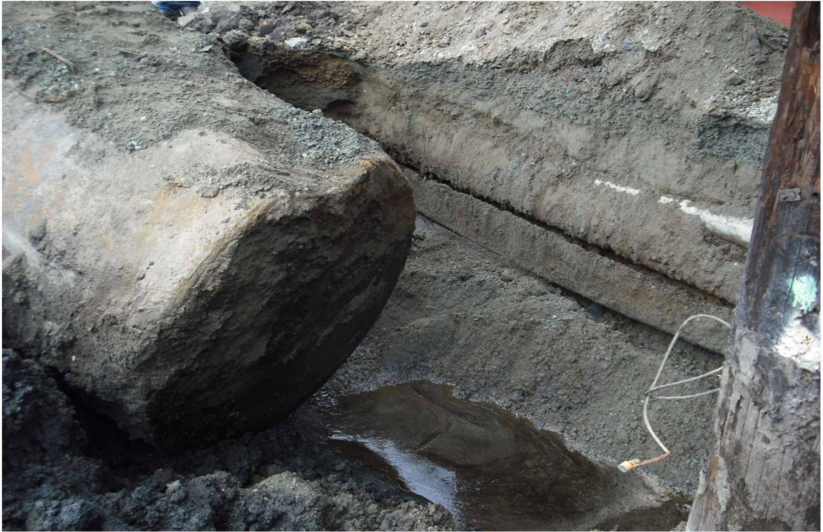
Oily water in UST pit
