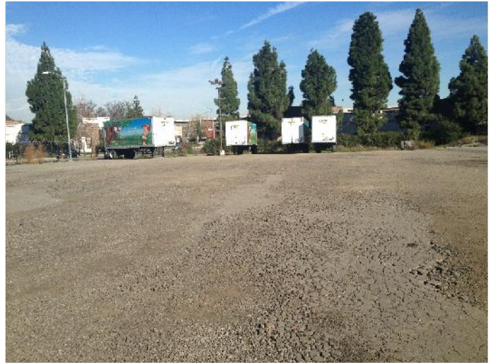
AN EXAMPLE OF THE CRACKED PAVEMENT AT THE SITE. TAKEN FROM THE MIDDLE OF THE SITE FACING EAST
