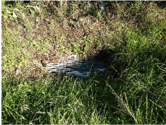
STORM DRAIN IN THE VEGETATED STRIP ONSITE
