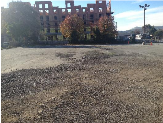
AN EXAMPLE OF THE CRACKED PAVEMENT AT THE SITE. TAKEN FROM THE MIDDLE OF THE SITE FACING WEST
