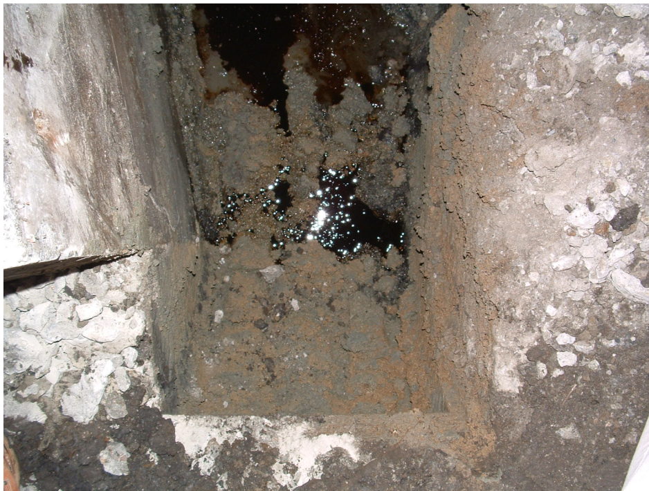
Fig. 1. Photograph of the hydraulic fluid released from the gravel zone around the ring roller foundation.
