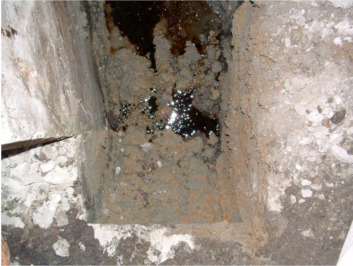
Figure 4. Oil seeping into the excavation near the NW corner of the roller pit.
