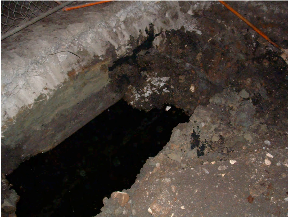
Figure 2. Oil seeping into the excavation from the top center of the photo.
