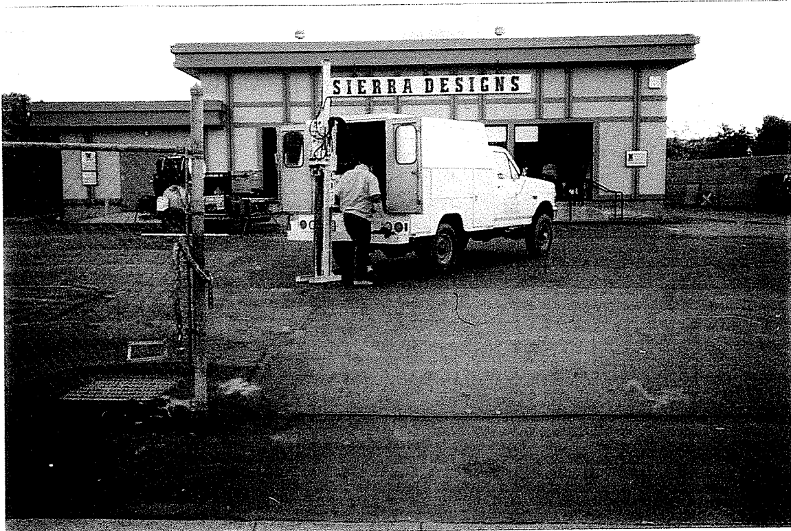
Photograph 2 View looking east at Geoprobe setup on SB-3, which was installed in the former UST excavation.
