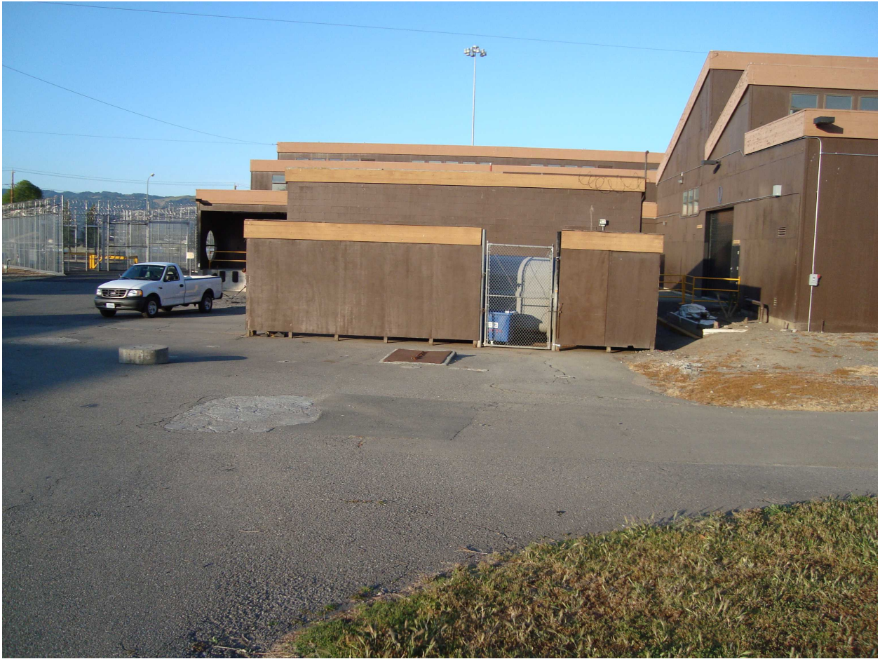
Photo 2: Generator Building behind chain link gate enclosure. Building Q to right, main gate to left. View is to west southwest.
