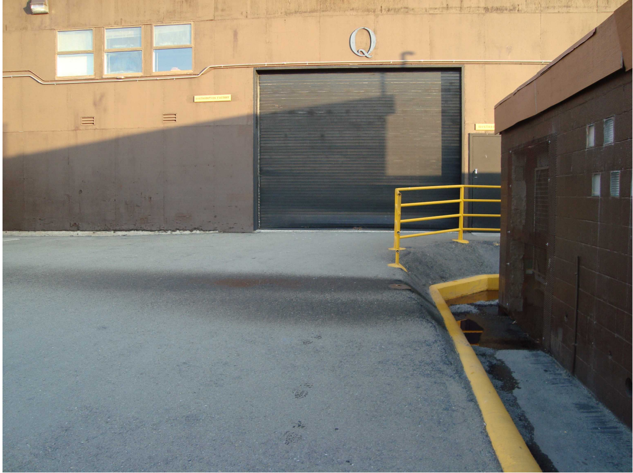
Photo 9: Building Q, south side; Generator Building is to left, showing walkway and low retaining wall. Fuel has flowed to the south along the wall. View is to the north.
