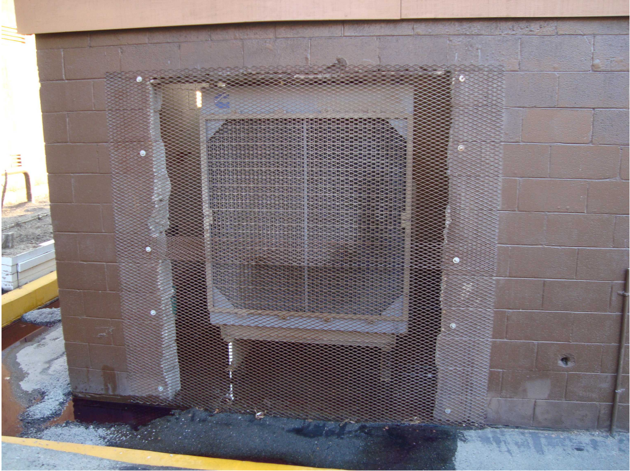
Photo 8: Generator Building, west side, fresh air ventilation wall penetration with screen in center of photo. Radiator of generator is visible through screen. View is to the east.
