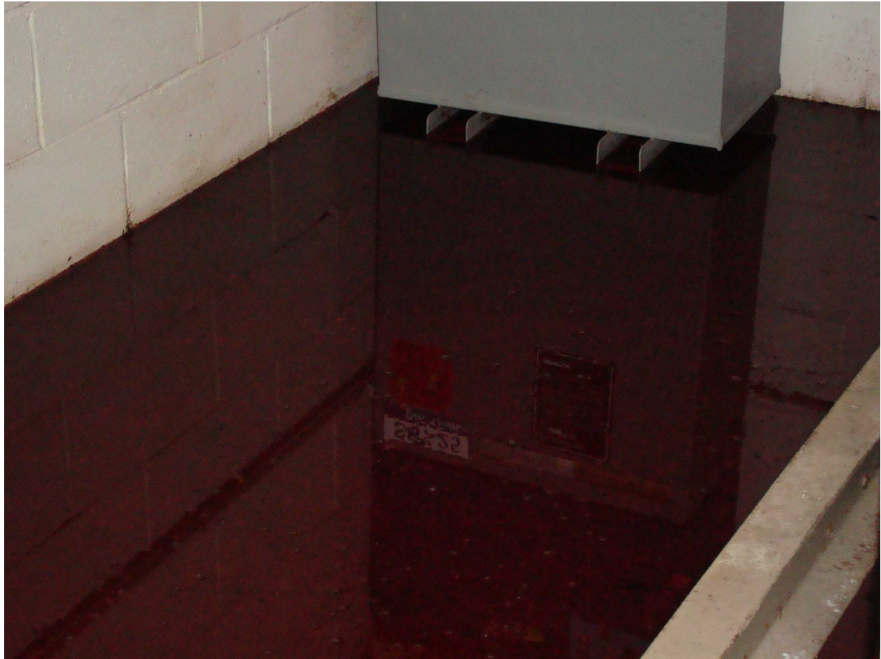
Photo 5: Generator Building floor showing shallow pool of fuel before deployment of absorbent.
