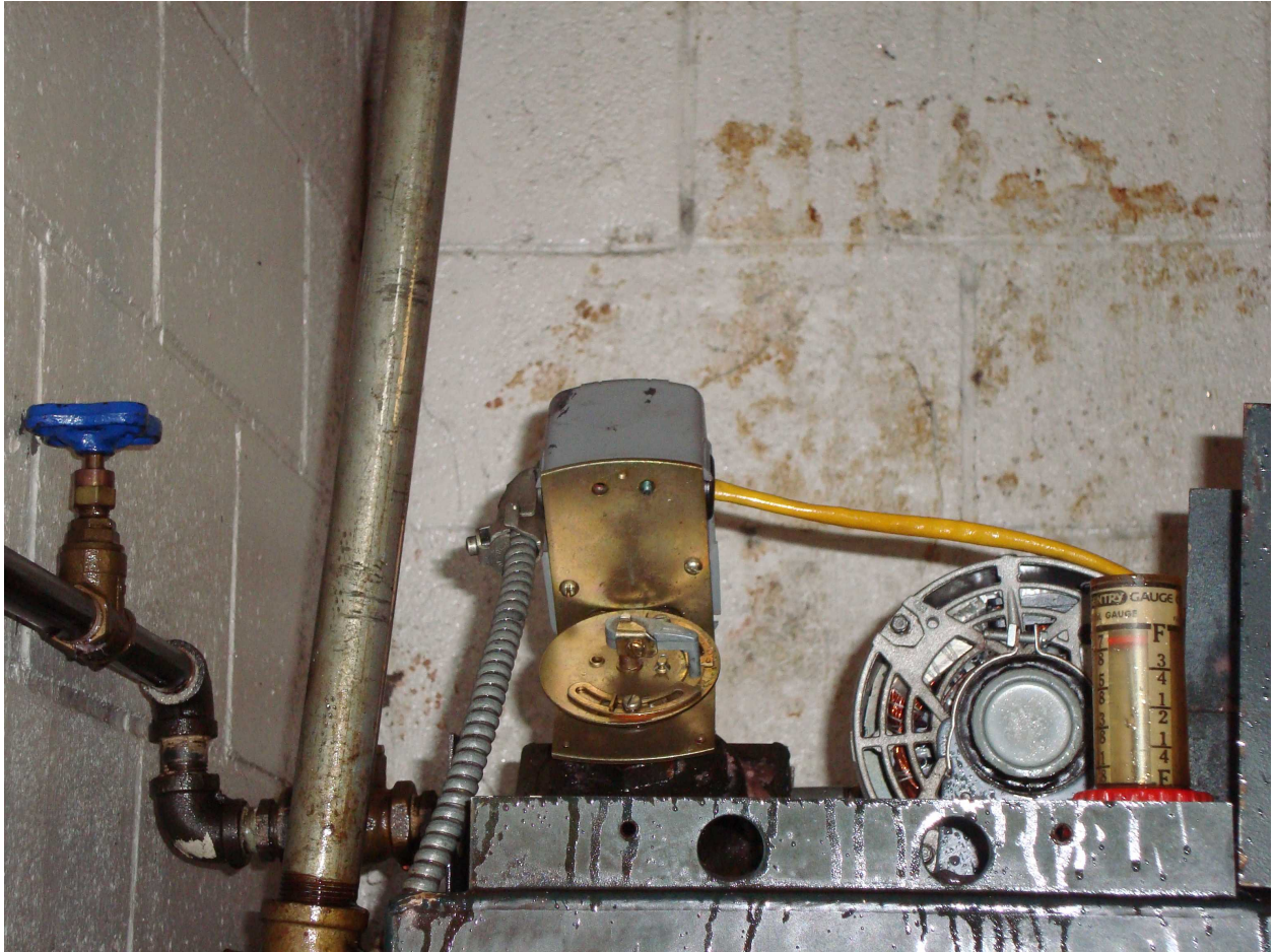
Photo 3: Day tank level sensor refill pump shutoff.
