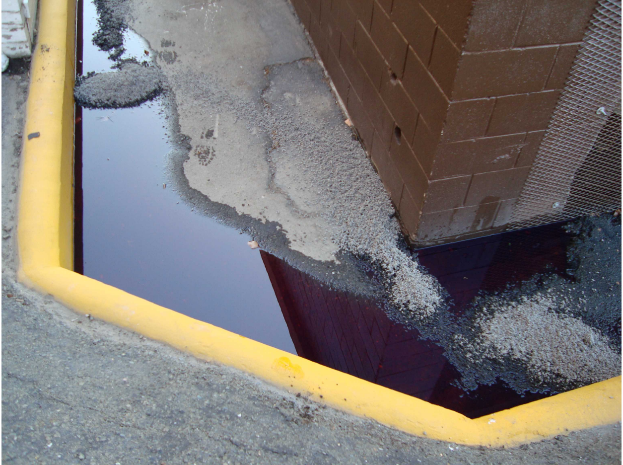
Photo 7: Generator Building, north side. Fuel collected against retaining wall. View is to the southeast.
