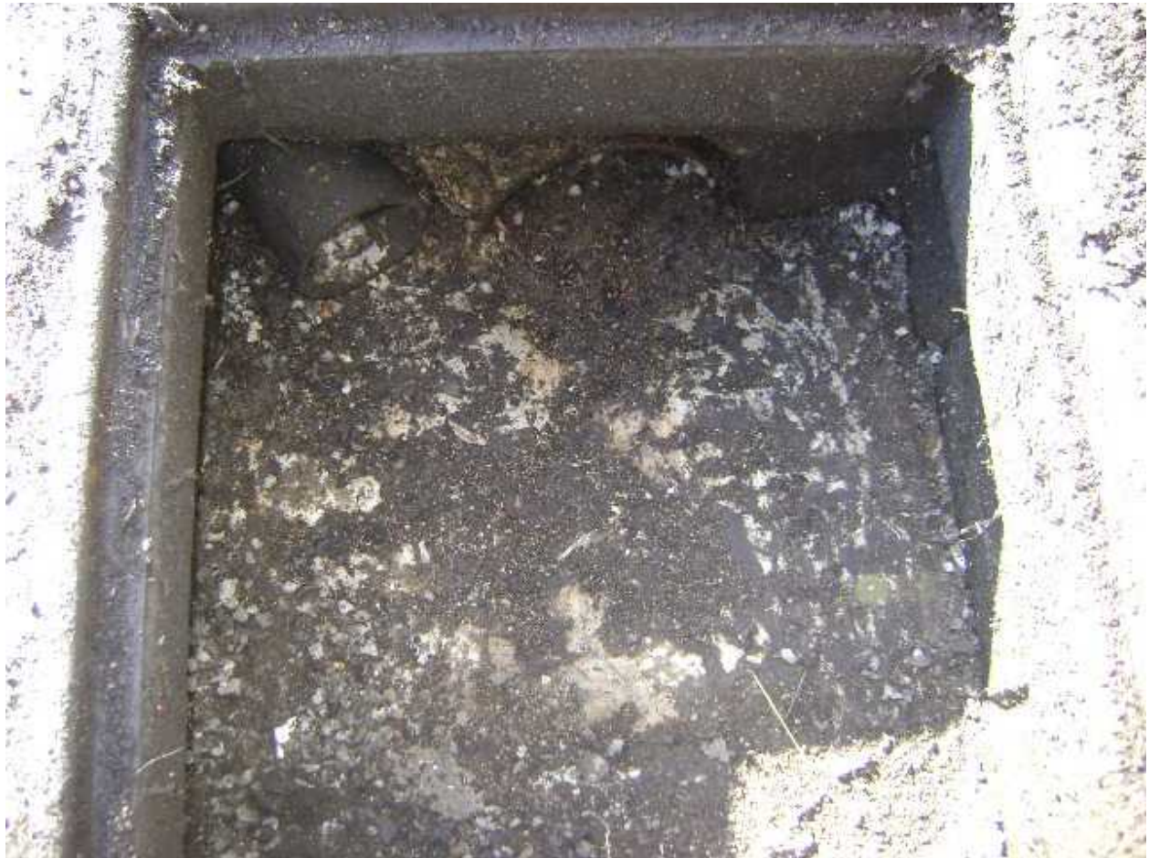
Photo 15: Dock well storm water catch basin detail. Pipe at top right corner conveys storm water from south trench segment to catch basin. Half-buried larger pipe at top center is catch basin connector to site storm water system. View is to south west.
