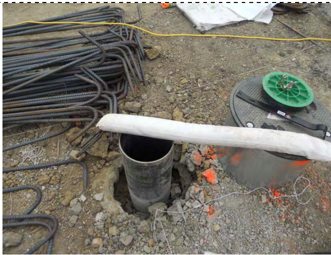
Photograph 3 - Material after about one hour in well on July 24, 2012.
