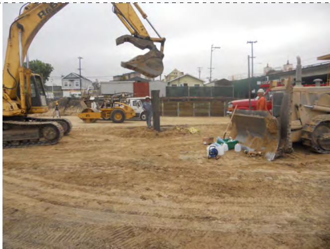
Photograph 5 - The 20-foot long pipe was driven into the subsurface using the excavator bucket.
