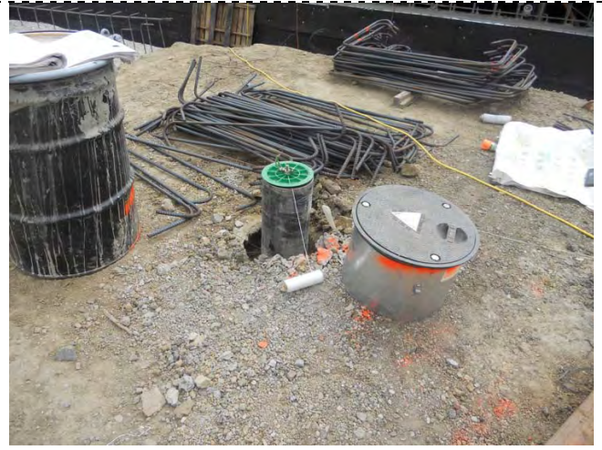
Photograph 2 - On July 24, 2012 the Geosorb was lowered into EW-2, note line connecting to the Geosorb
