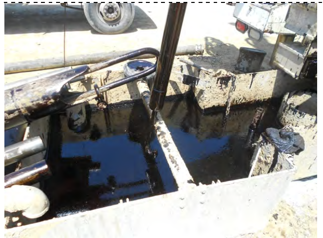
Photograph 10 - View of the catch basin.
