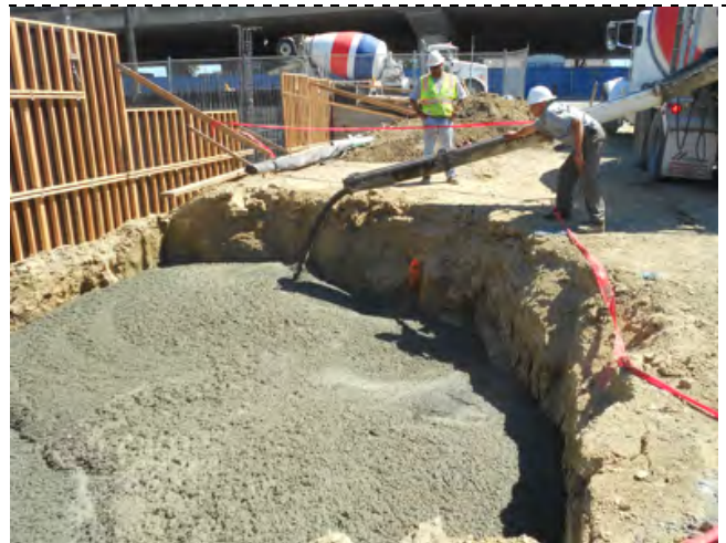
Photograph 24 - The second to the last load of concrete slurry filling excavation to near the bottom of proposed footings.
