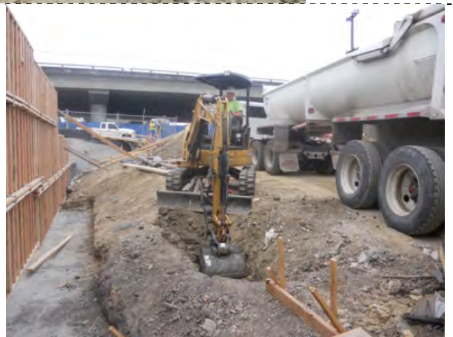
Photograph 12 - Initial soil removal using small excavator with soil going directly into adjacent truck for delivery to Class II landfill.
