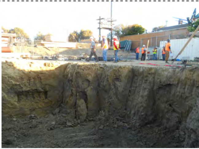
Photograph 19 - Expanding excavation became a safety hazard.
