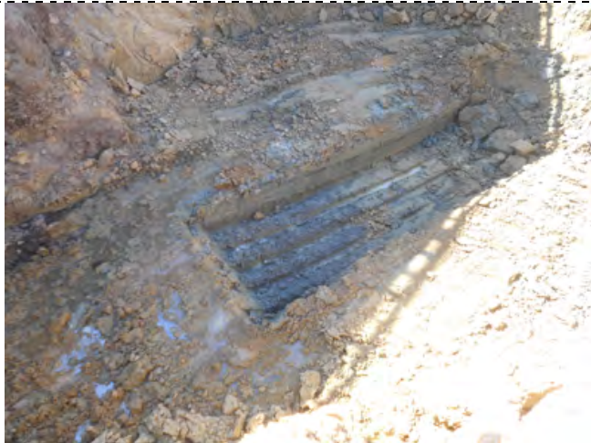
Photograph 21 - Once the width and breadth of the excavation became a safety hazard and attempt was made to find the bottom of contamination by digging a trench in the middle of the pit.
