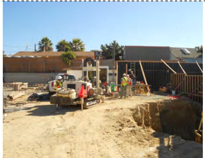
Photograph 20 - CPT and MIP rigs were conducting drilling operations at the same time that the tank pit was being over-excavated.
