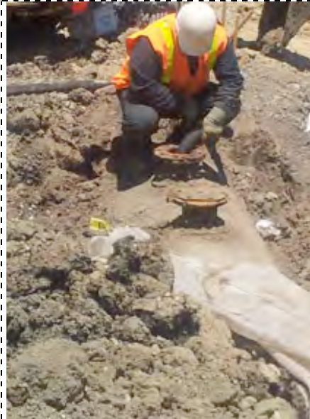
Photograph 4 . Removing water from tank, which was placed directly into a vacuum truck.
