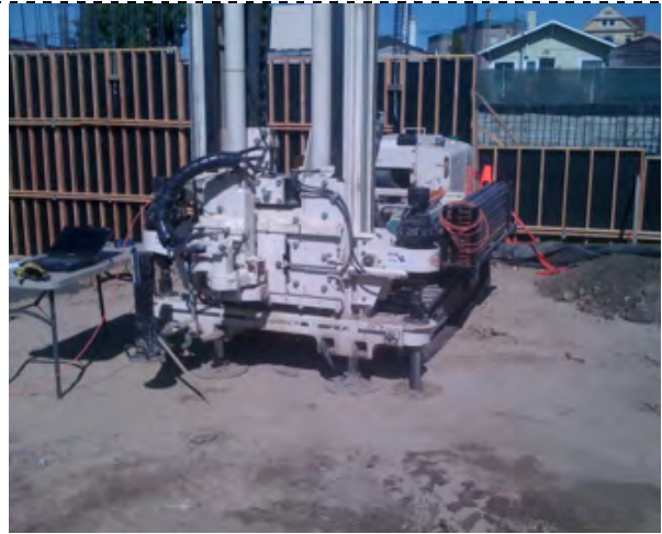
Photograph 2 - CPT rig over MIP-6, view east. This became the location of EW-2.
