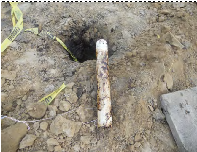
Photograph 3 - A 4-inch diameter Teflon bailer was initially used in an attempt to remove free product. The layer was found to be very thin.
