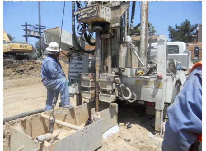
Photograph 8 - It was necessary to drill through two well encumbrances prior to adding slurry and removing water.
