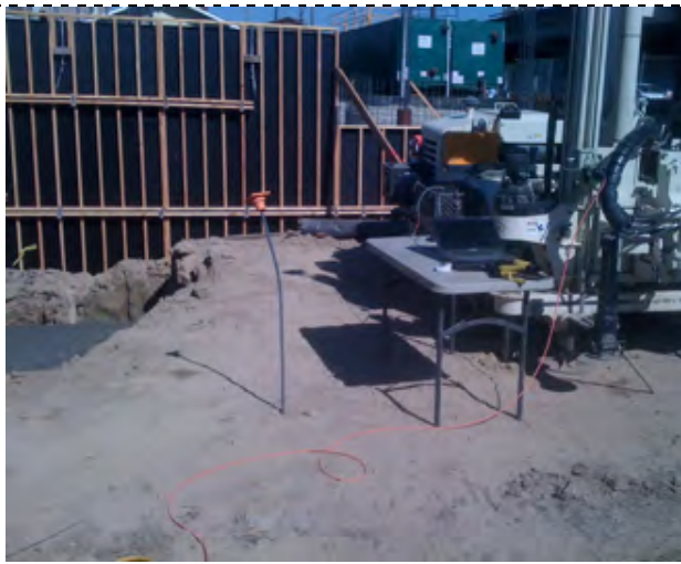
Photograph 3 - CPT rig (Geoprobe 6625), note UST #4 excavation with CDF to left of rig.
