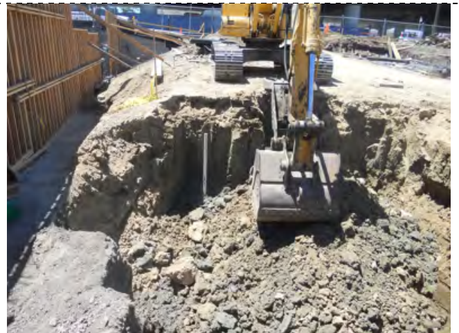
Photograph 18 - PVC pipe on left center of photograph is MW-3 installed by Kleinfelder and abandoned by Fugro.
