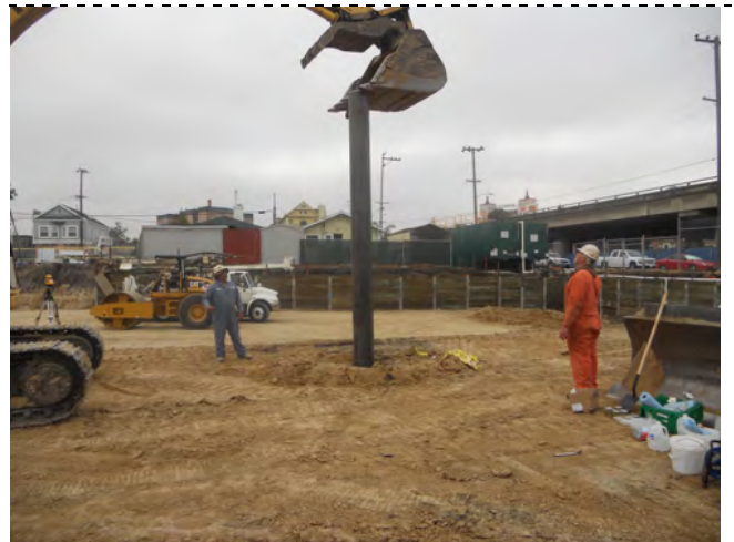
Photograph 4 . Pitcher Drilling forced a larger diameter pipe over the well casing to facilitate proper removal of the water in the well.
