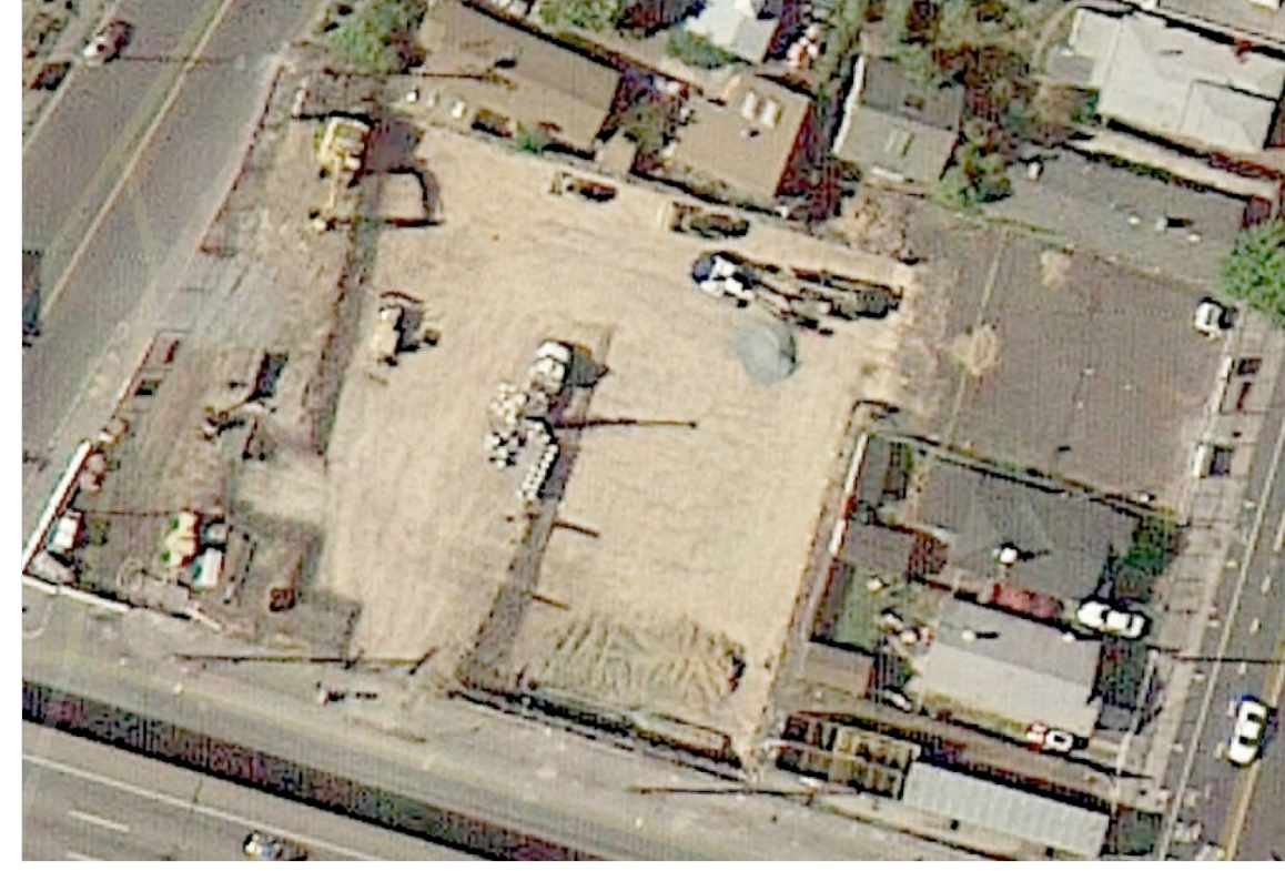
Photo 3 Google Earth image of the Property during abandonment of the 1905 production well. Image date is May 20, 2012. At grade confirmation soil samples were collected May 15, 2012, five days previous to this image.
