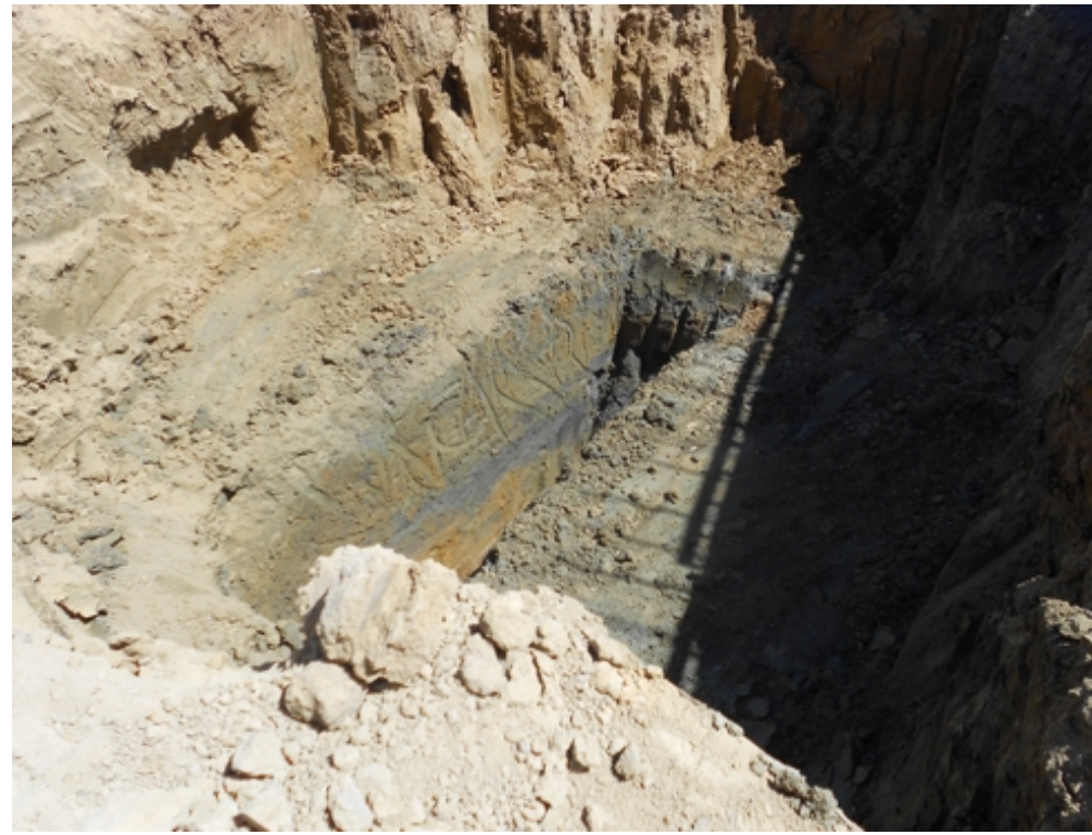
Photo 2 UST 4 -The trench at the bottom of the excavation is five feet deep and as wide as the bucket on the backhoe. The top of the trench is about eight feet below the top of the excavation, which is about five feet below original ground surface. The trench remained open for about 90 minutes while groundwater seeped in at a ver slow rate. One liter of water was collected from the bottom of the trench prior to filling the excavation with a concrete slurry due to safety concerns for onsite workers and equipment.
