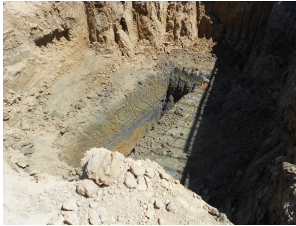
Photo 2 UST 4 -The trench at the bottom of the excavation is five feet deep and as wide as the bucket on the backhoe. The top of the trench is about eight feet below the top of the excavation, which is about five feet below original ground surface. The trench remained open for about 90 minutes while groundwater seeped in at a ver slow rate. One liter of water was collected from the bottom of the trench prior to filling the excavation with a concrete slurry due to safety concerns for onsite workers and equipment.
