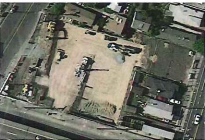
Photo 3 Google Earth image of the Property during abandonment of the 1995 production well. Image date is May 20, 2012. Air grade confirmation soil samples were collected May 15, 2012, five days previous to this image.
