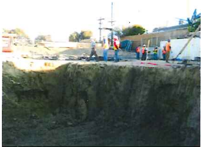
Photo 1 UST 4 - over excavation. Decision was made to stop excavating the width and breadth due to safety concerns. A five-foot deep trench was excavated at the bottom of the excavation, as shown below, in an attempt to remove as much contaminated soil as practical within safety constraints.
