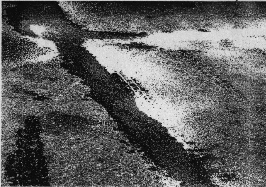
Spill in driveway not cleaned up
