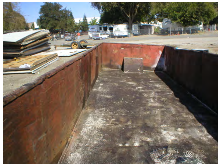
Photo 4. Rolloff Bin condition prior to removal from site
