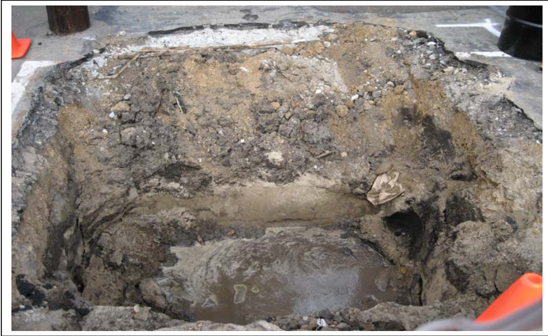
Photograph 9 – Water in Bottom of UST #4 Excavation
