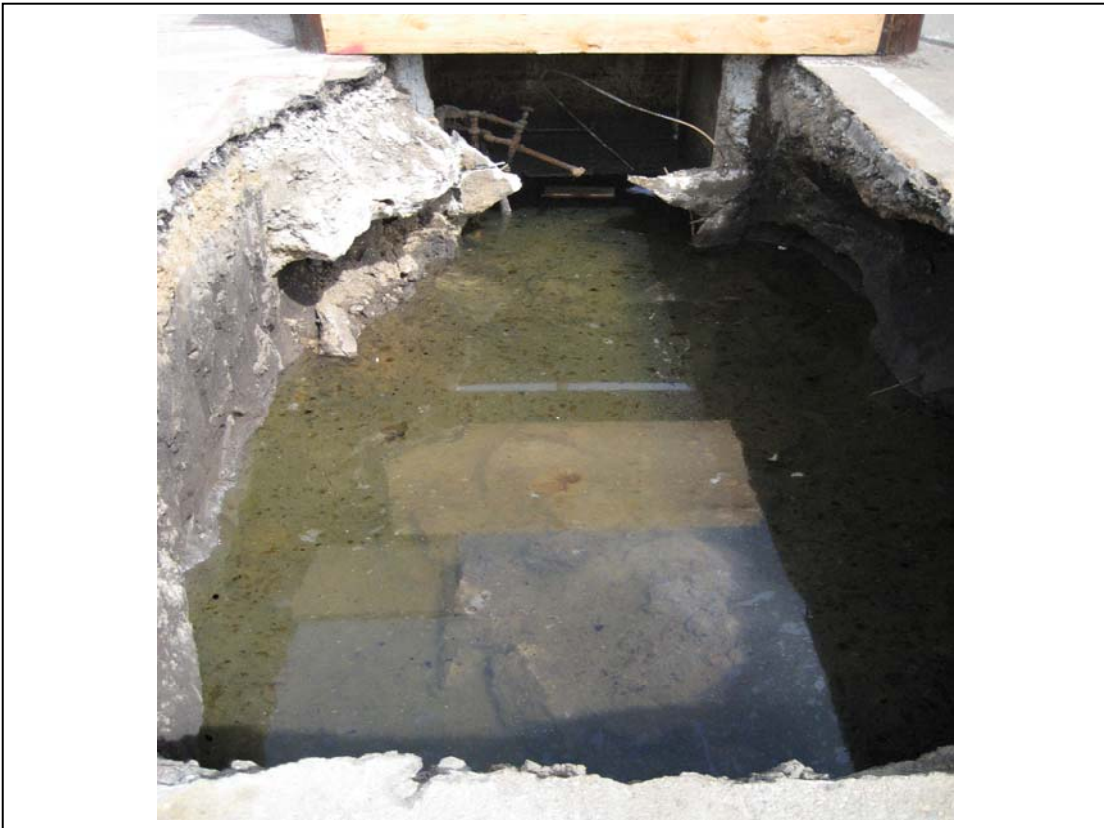
Photograph 10 – Water in Bottom of UST #2 Excavation
