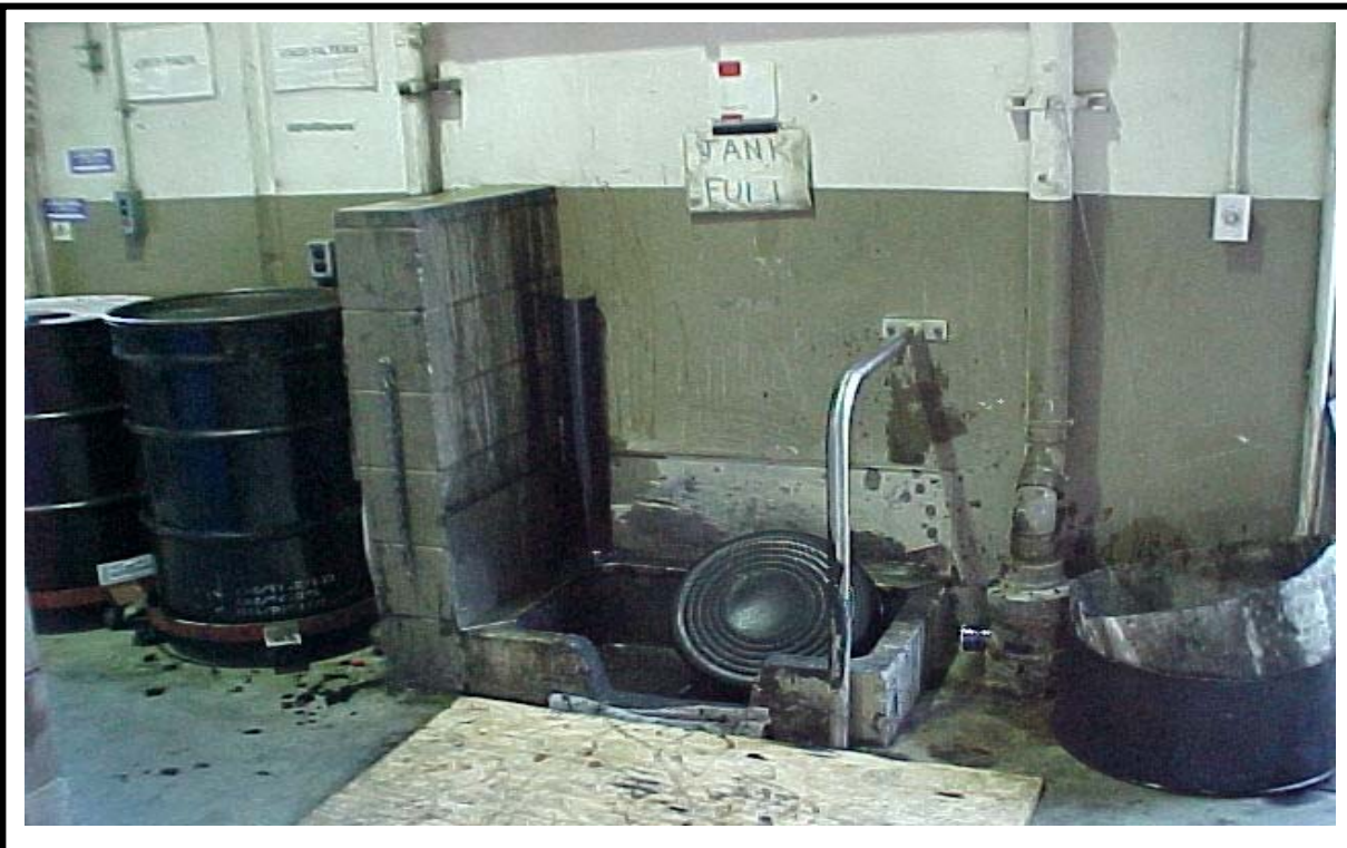
Photograph 1: Original Remote Waste Oil Drain
