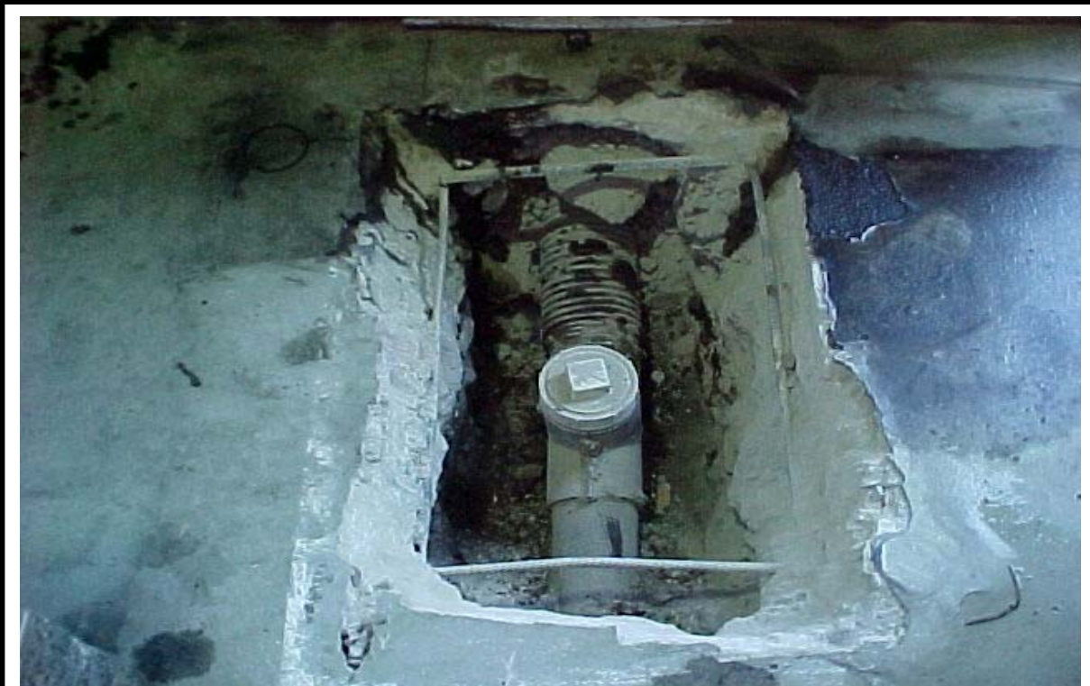
Photograph 2: Piping Cleanout to Remote Waste Oil Drain
