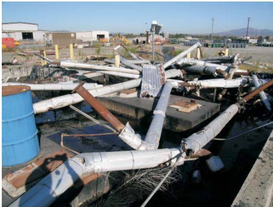
Piping in Containment Structure
