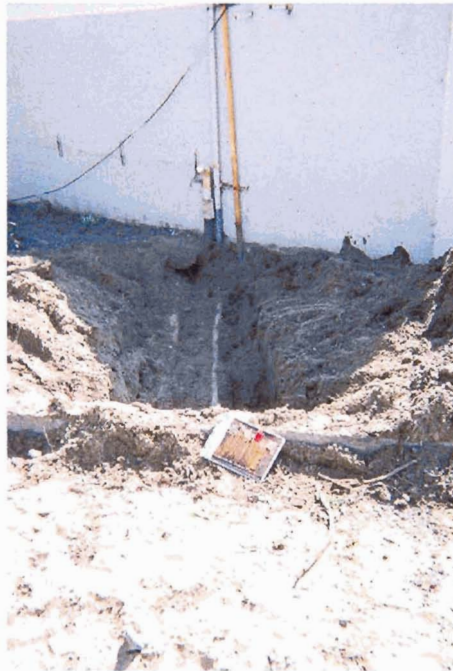
Photo 6 – View southeast of the supply and vent line pit. Foreground clipboard for scale.
