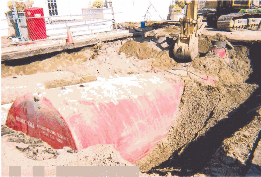
Photo 1 – Exposed gasoline UST at Grand Marina.
