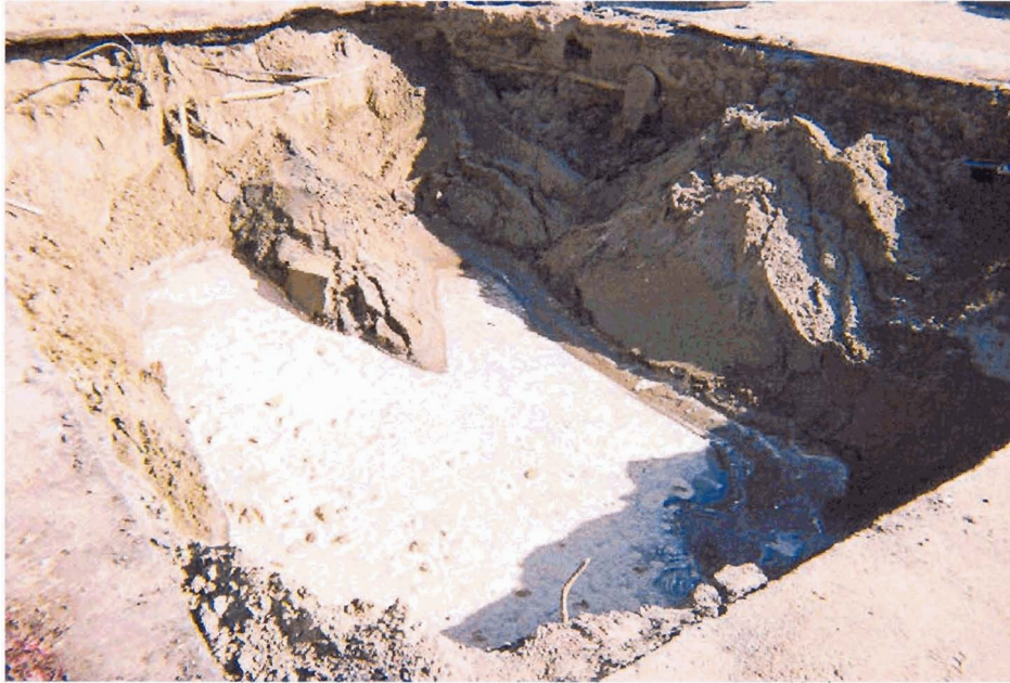
Photo 5 - View southeast of water in the bottom of the UST excavation pit.
