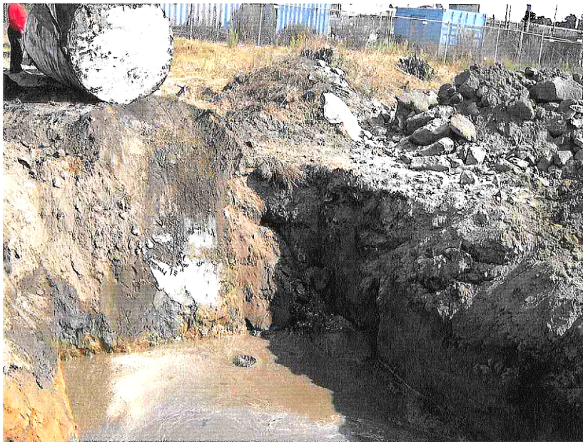
Photograph 2 – Looking at tank excavation pit with groundwater. Note discolored soil that was eventually overexcavated and removed.
