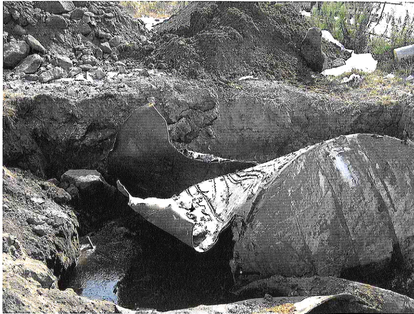
Photograph 1 – Looking at cut opened 3,000-gallon tank and stockpiles of tank contents (concrete slurry) and excavated soil.
